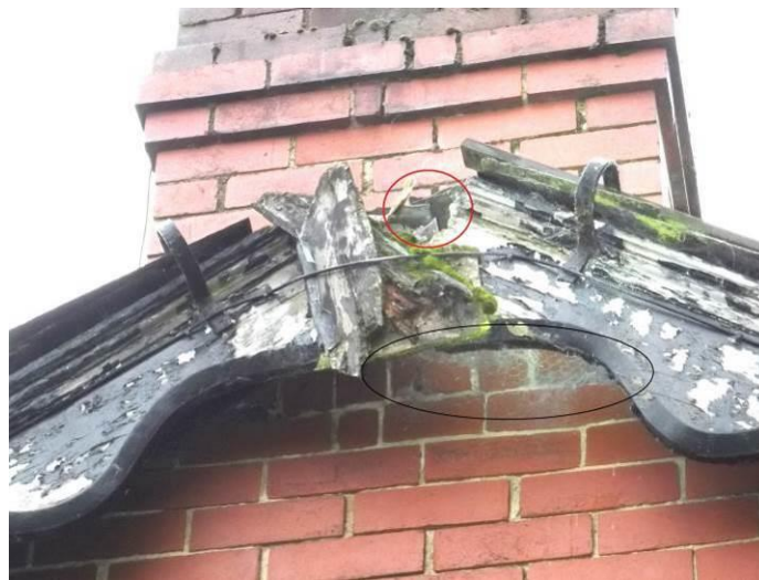
Possible bat access circled in red, mesh circled in black
