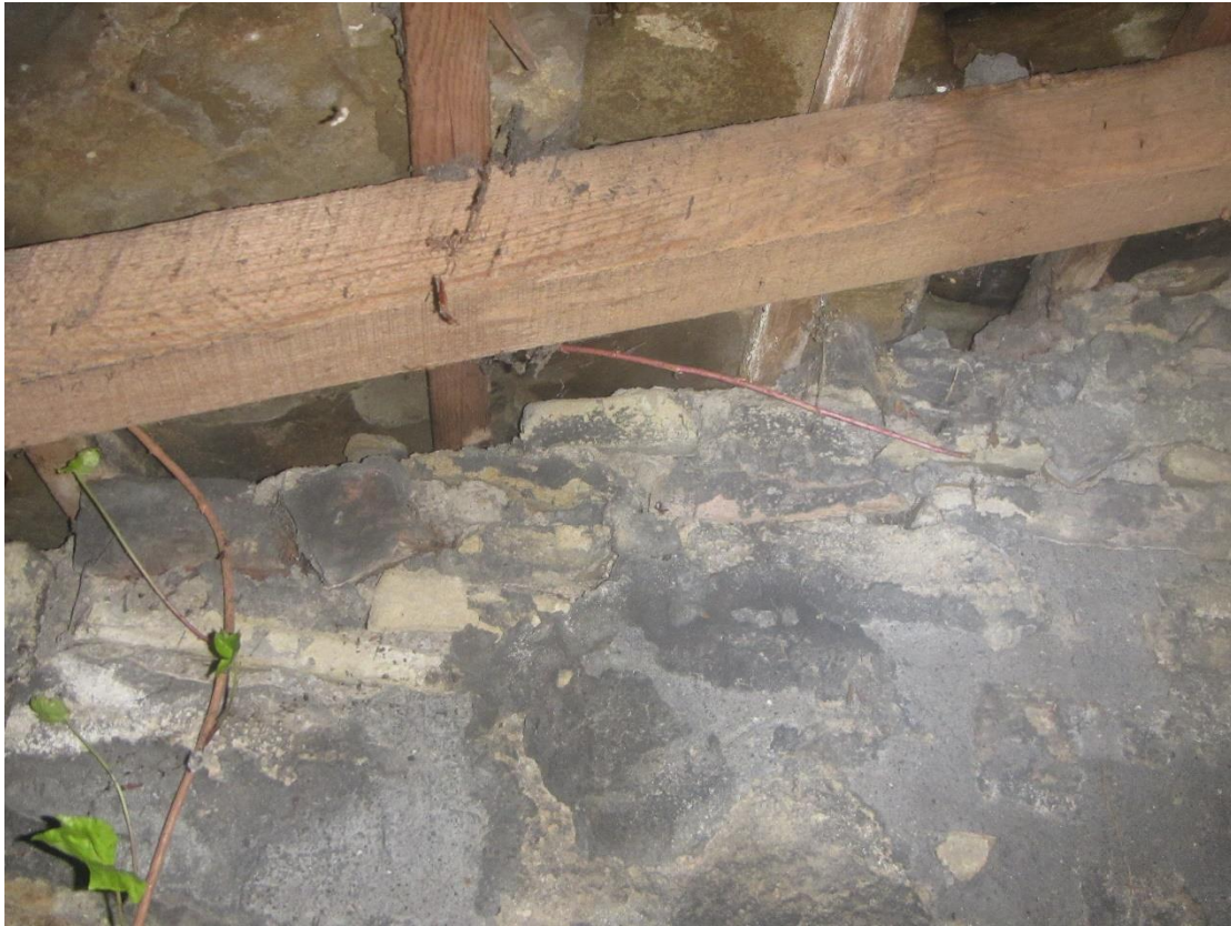
Photograph 19 – Example gaps above the wall plate within Building 1.
