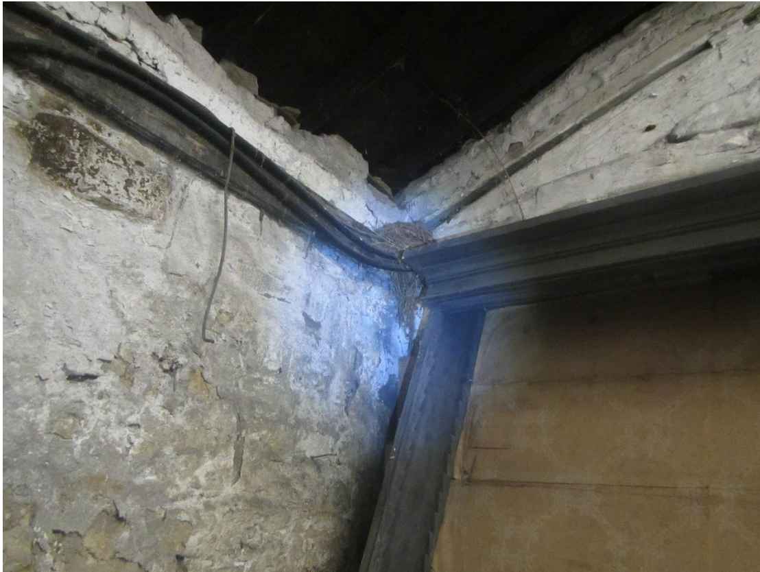
Photograph 23 – Birds nest located within Section A of Building 2.
