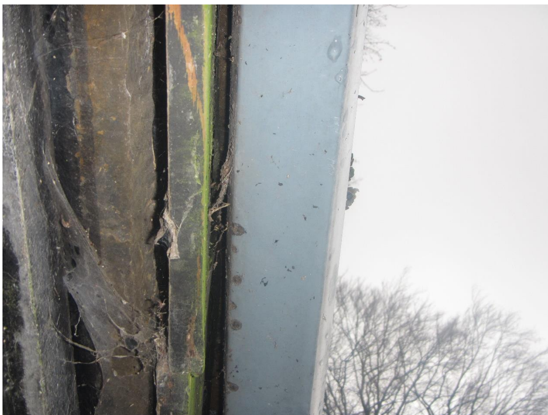
Photograph 17 – Gap between the wooden barge board and the wall on Building 4.
