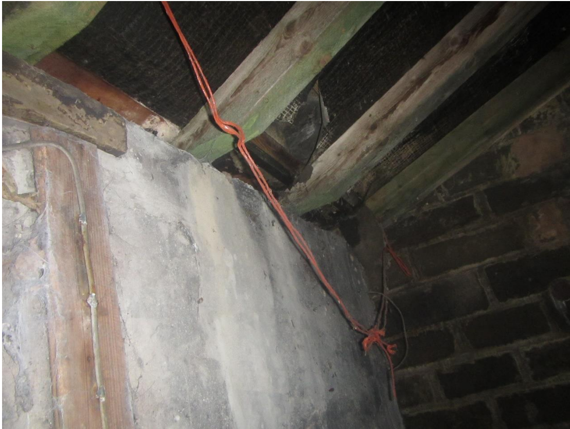
Photograph 31 – Internal view within Building 4, gaps above the wall plate.
