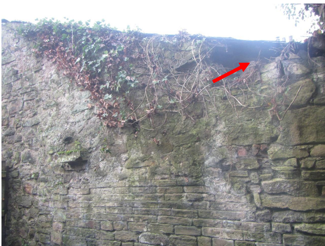
Photograph 8 – The northern aspect of Building 2, view of large gap below tiles where stonework is missing. Arrow pointing to location of a historic bird's nest.
