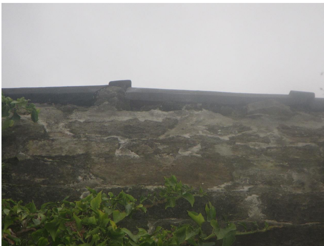
Photograph 6 – Gaps where mortar is missing underneath the ridge tiles on Building 2.
