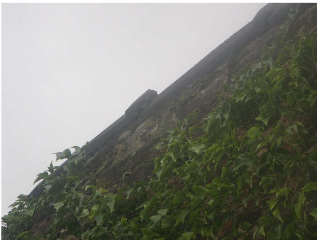
Photograph 7 – Example gap on the ridge tile on Building 2 where mortar is missing.
