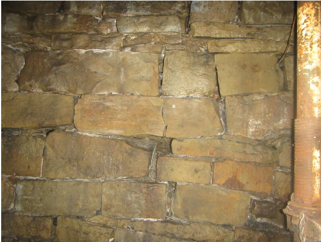
Photograph 29 – Gaps in the stonework within Building 3.
