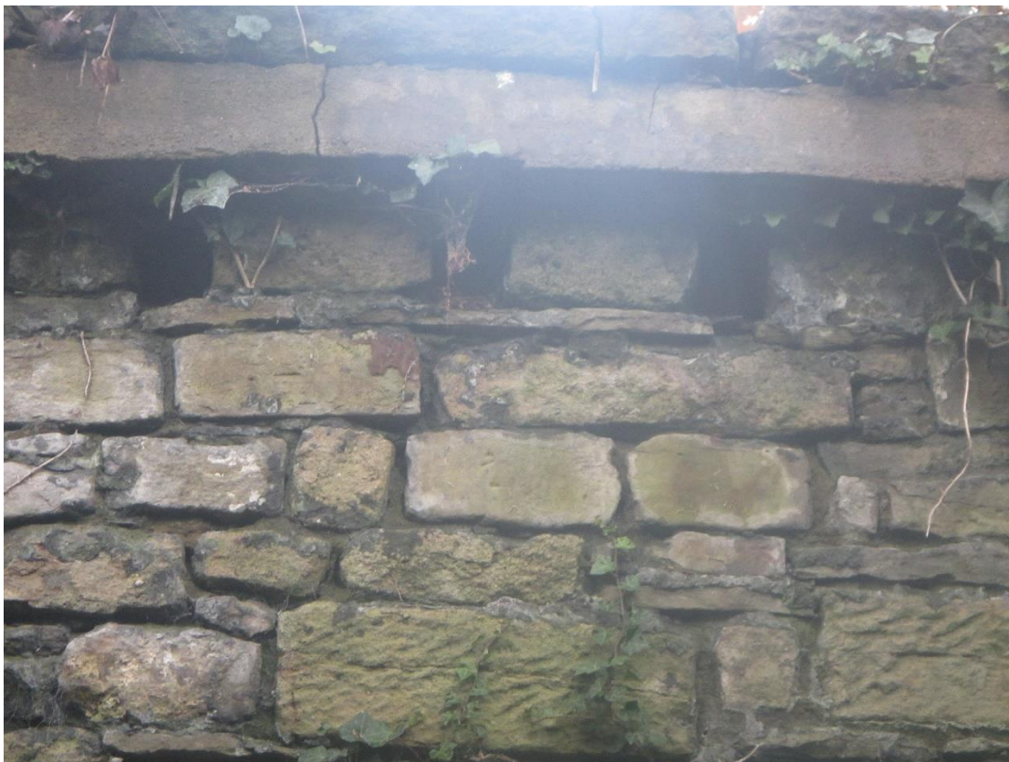
Photograph 14 – Close view of the large gaps at the apex of the wall on the eastern aspect of Building 3.
