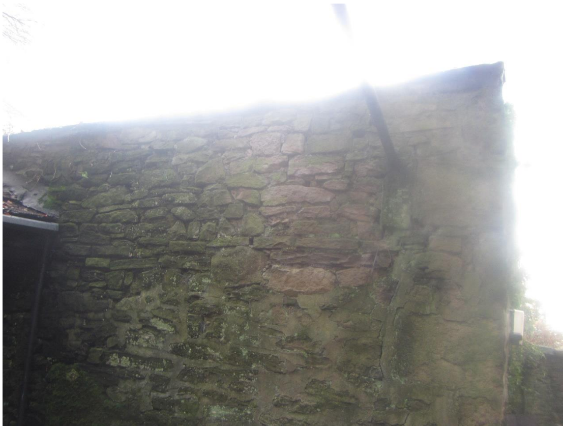
Photograph 9 – Western aspect of Building 2, with several superficial gaps in the stonework.
