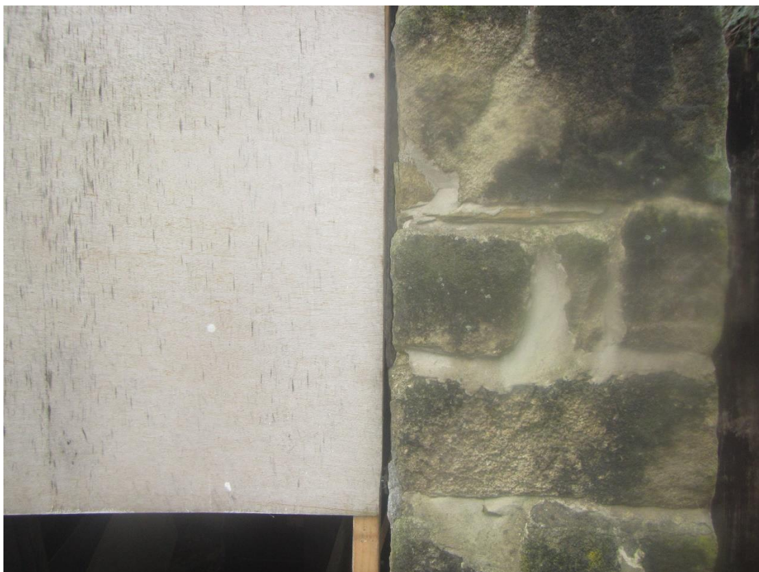
Photograph 10 – Gaps between the stone and MDF boarding on the eastern aspect of Building 2.
