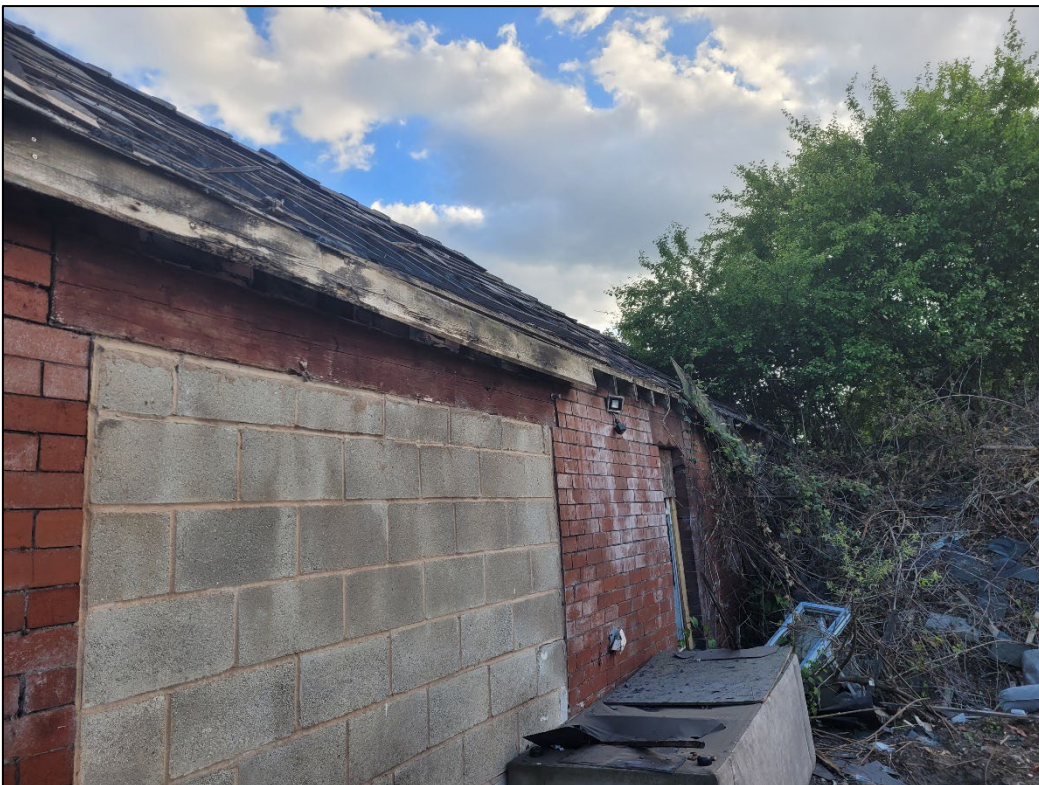
Photograph 2 Gaps on the underside of eaves and between fascia boards and top bricks
