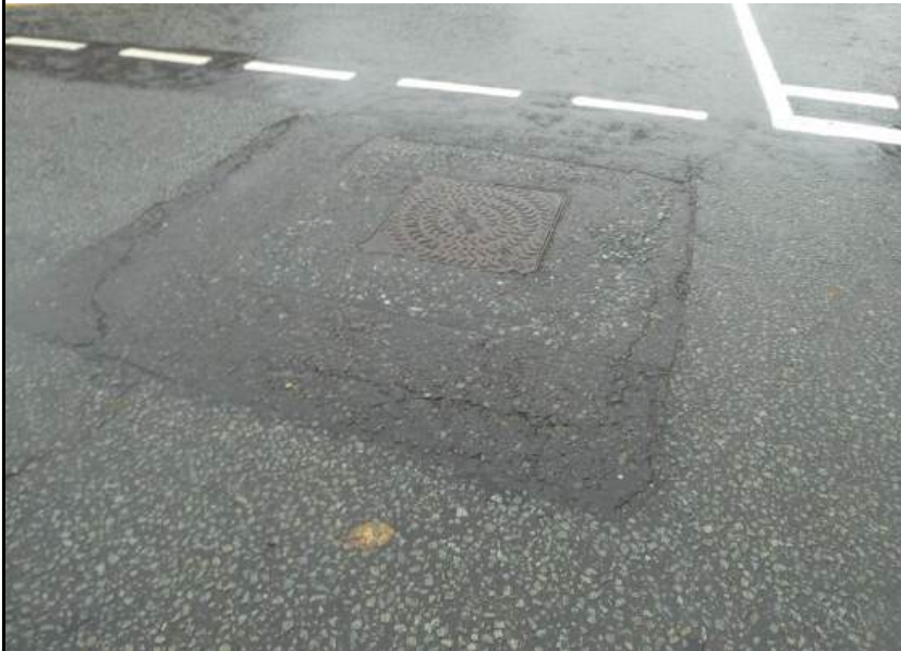
Photograph 51. Cracking and erosion to surfacing.
