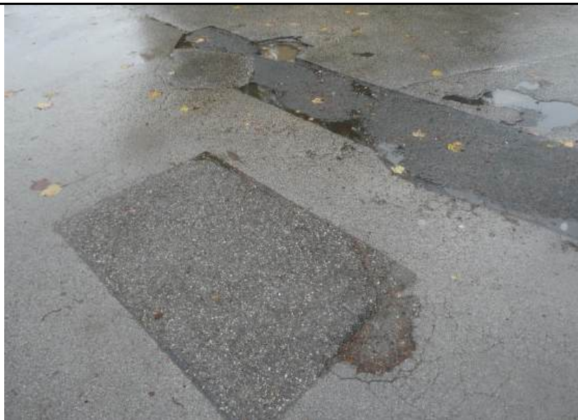
Photograph 26. Reinstated area of surfacing damaged and eroded
