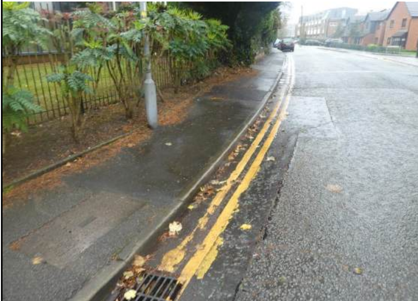
Photograph 35. Line marking eroding
