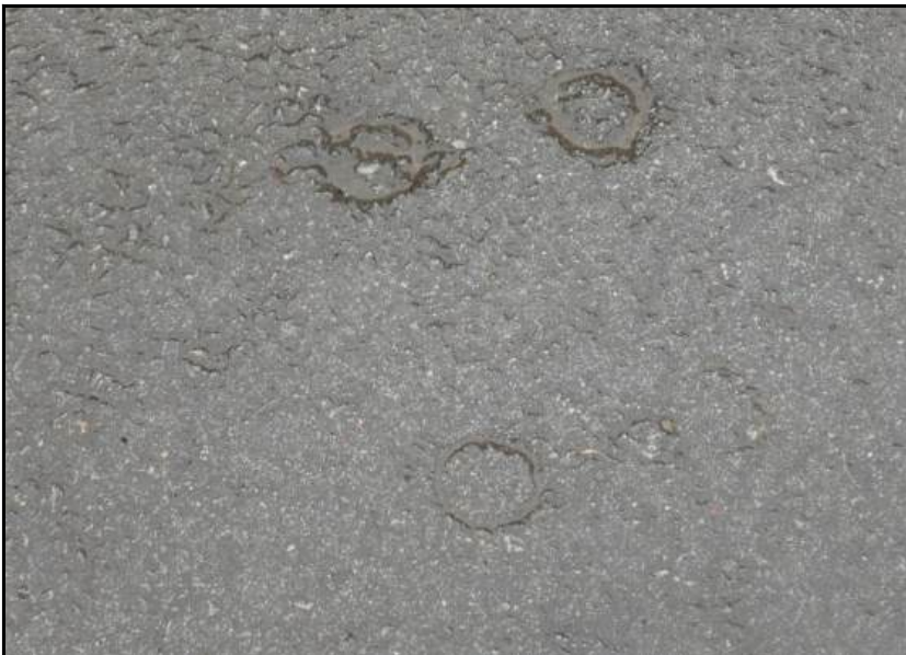
Photograph 9. Localised indentations to footpath areas
