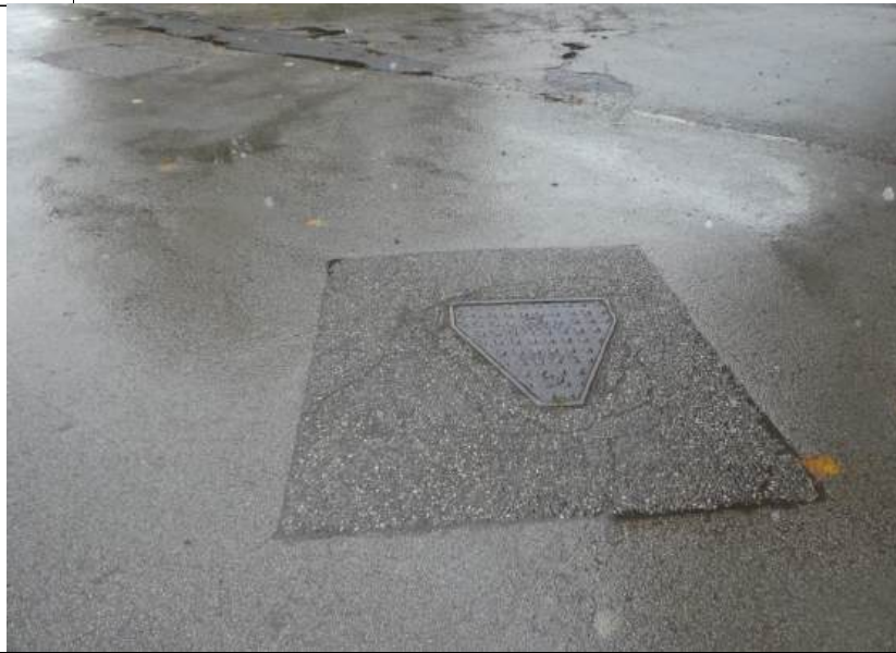
Photograph 24. Reinstatement to inspection chamber cracked and eroding
