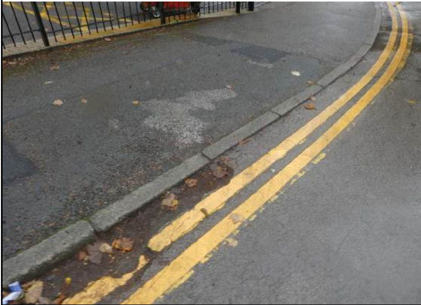
Photograph 23. Uneven and damaged kerb to George Street
