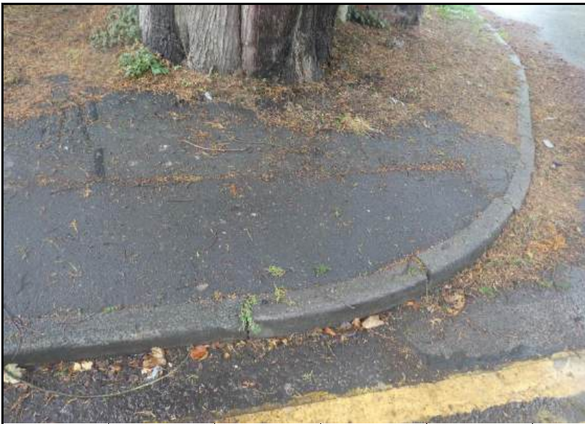
Photograph 41. Damaged and uneven kerbing.
