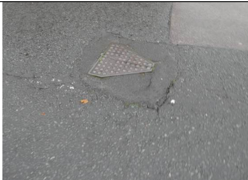
Photograph 86. Erosion to surfacing around inspection chamber.
