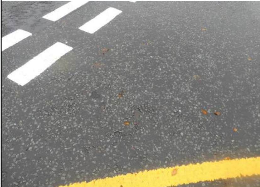
Photograph 11. Minor erosion to the surfacing at the junction with George Street.
