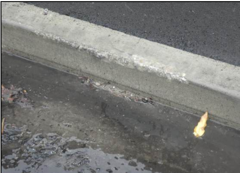
Photograph 5. Localised impact damage to the kerbs
