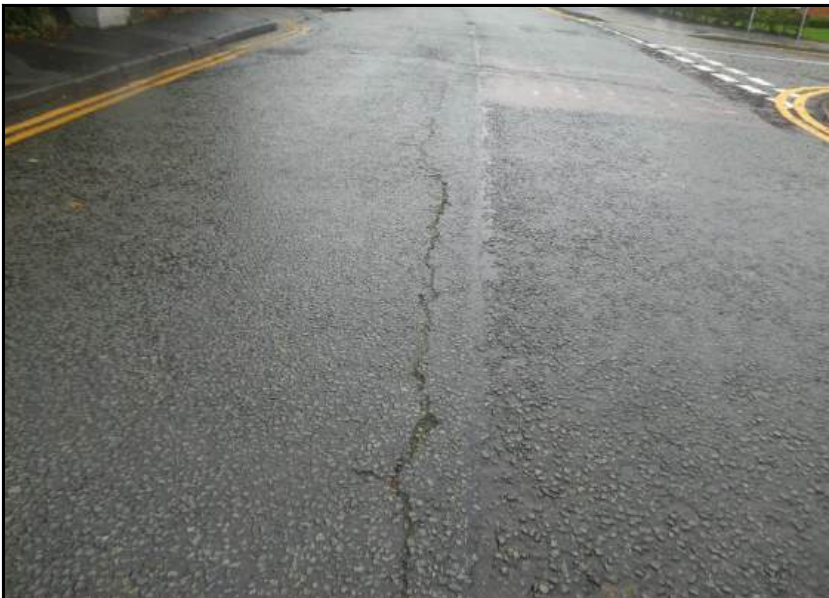
Photograph 45. Cracking to surfacing to centre of roadway.
