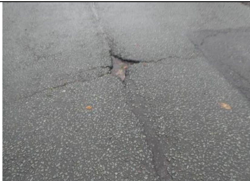
Photograph 50. Cracking and erosion to surfacing.
