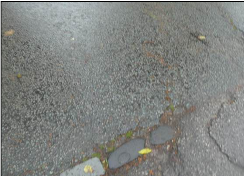
Photograph 33. Localised erosion to surfacing
