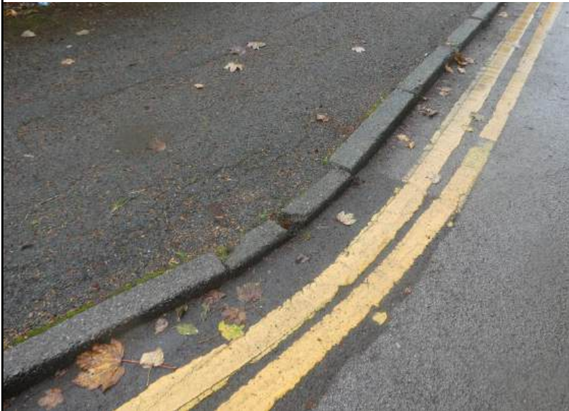
Photograph 19. Damaged and uneven kerbs to Norwood junction
