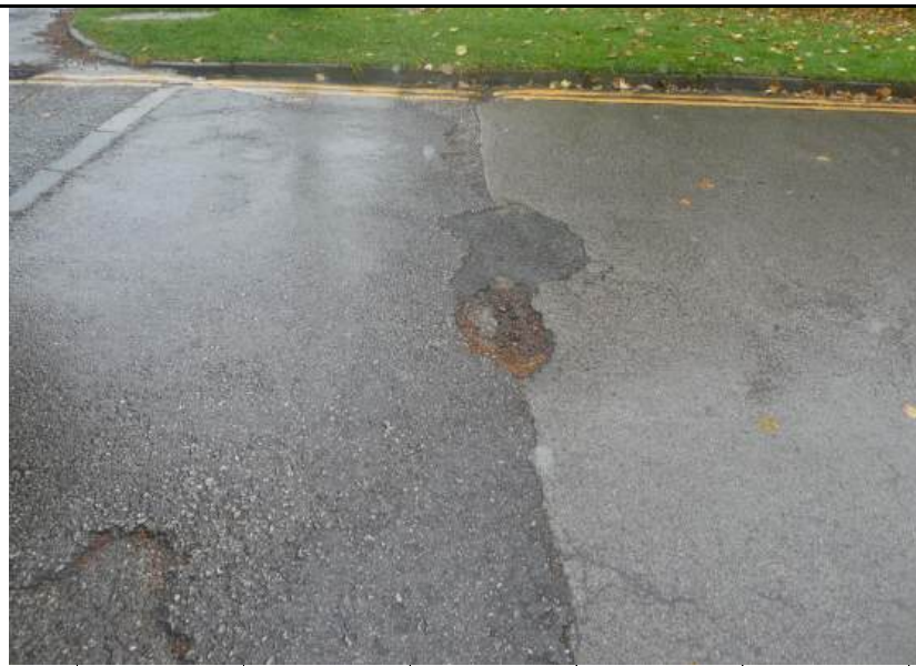
Photograph 30. Localised erosion to surfacing
