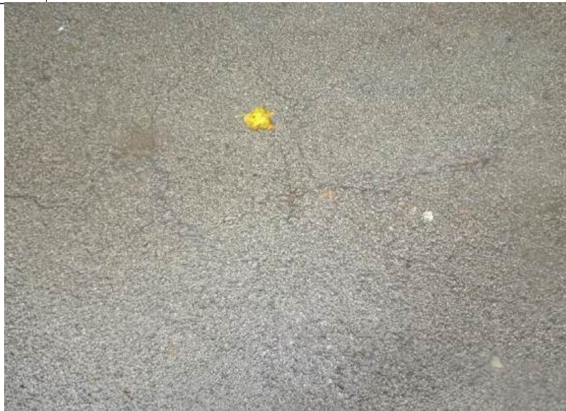
Photograph 20. Localised cracking to road surface
