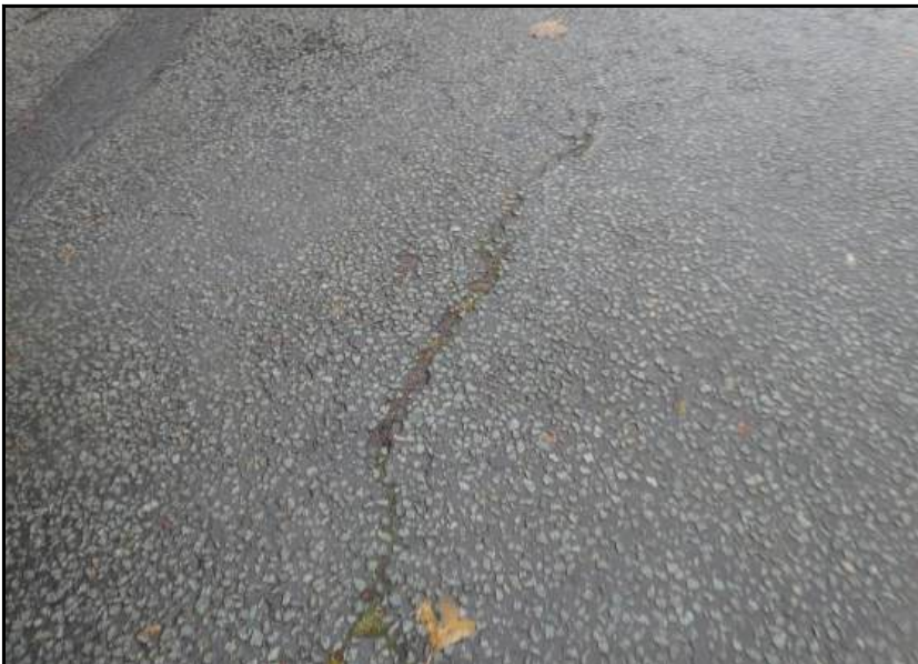
Photograph 49. Cracking and erosion to surfacing.
