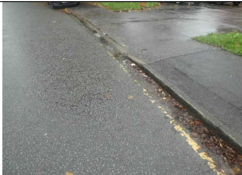
Photograph 70. Erosion to footpath
