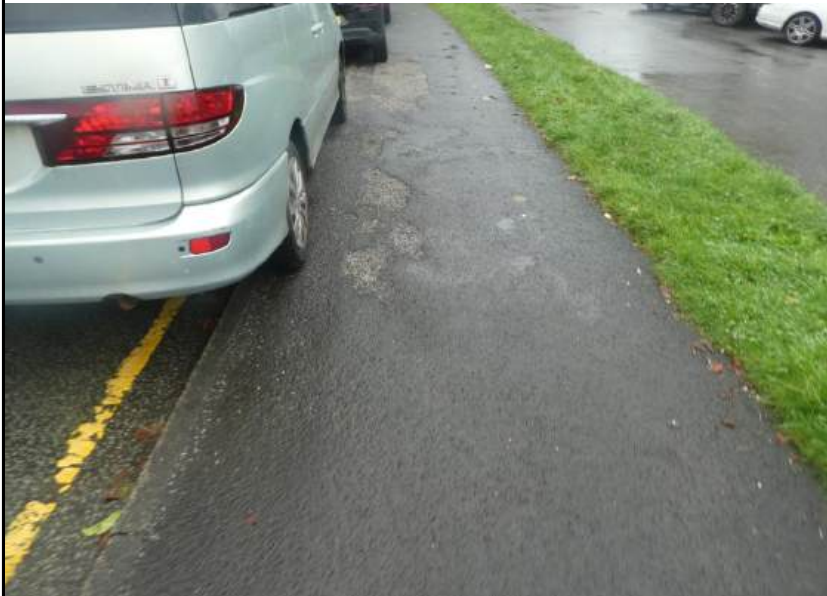
Photograph 67. Erosion to footpath
