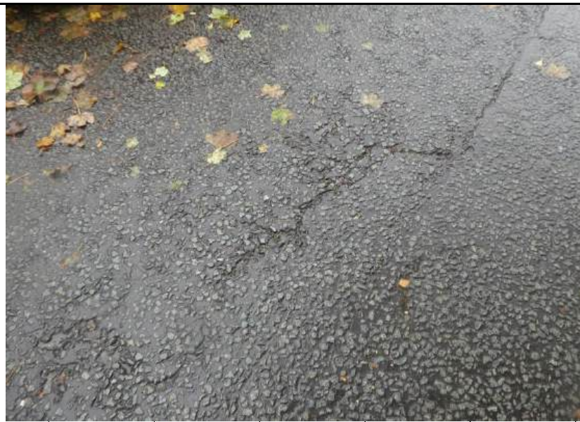
Photograph 78. Localised cracking to surfacing.
