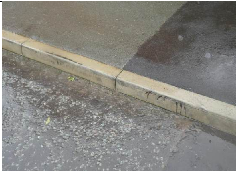
Photograph 8. Staining to the kerbing
