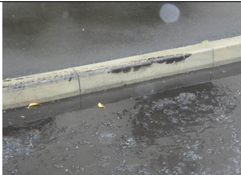
Photograph 6. Staining the kerbing
