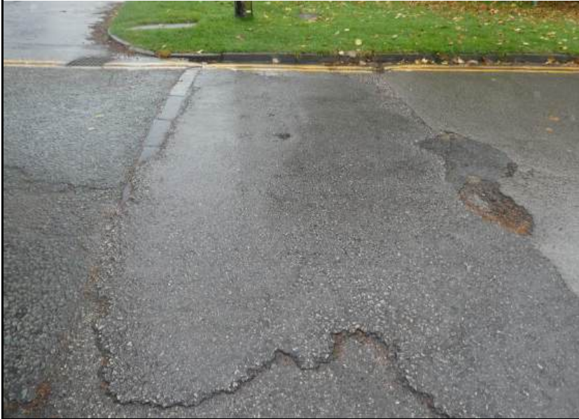
Photograph 31. Localised erosion to surfacing
