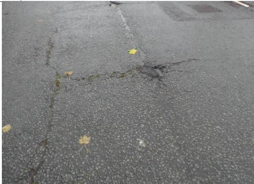
Photograph 48. Cracking and erosion to surfacing.
