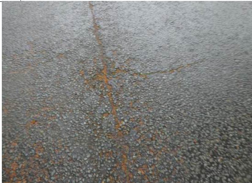
Photograph 40. Badly eroded and cracked surfacing.
