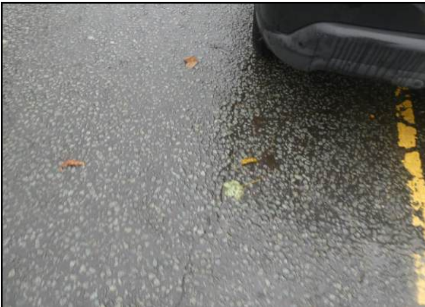
Photograph 69. Cracking to surfacing
