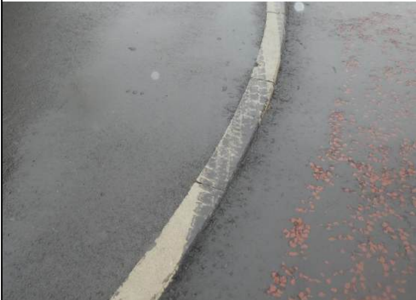
Photograph 3. Kerbing is stained and marked on both sides of the roadway
