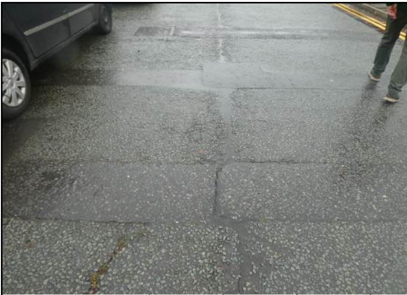
Photograph 53. Cracking to surfacing
