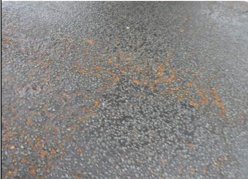
Photograph 39. Badly eroded and cracked surfacing.
