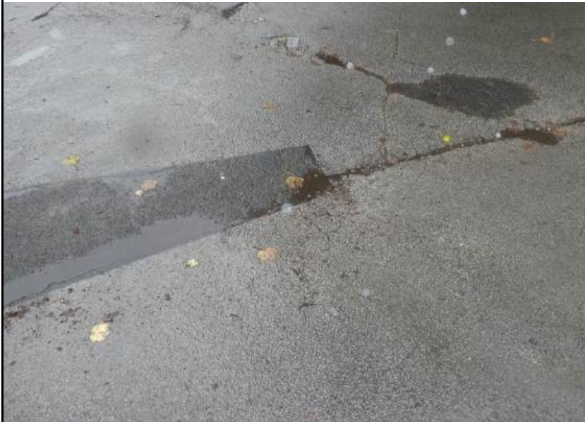
Photograph 27. Reinstated area of surfacing damaged and eroded
