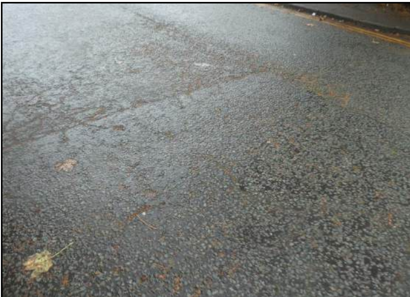
Photograph 37. Erosion of wearing coat of surfacing
