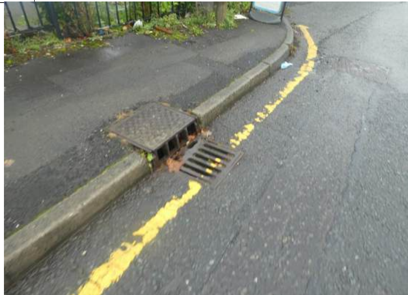
Photograph 88. Erosion to line marking.
