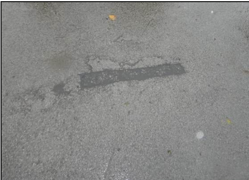
Photograph 25. Localised erosion to surfacing
