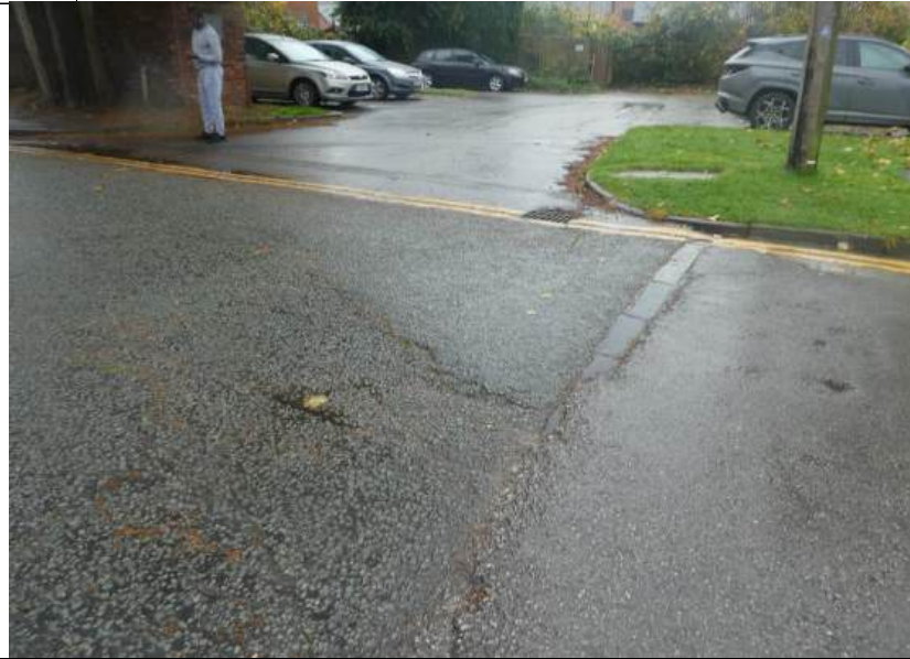
Photograph 32. Erosion to road surfacing near to site entrance on George Street
