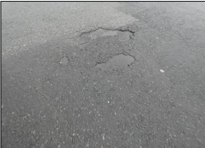
Photograph 89. Localised erosion to surfacing
