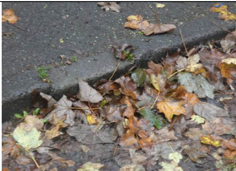
Photograph 74. Uneven kerbs to footpath
