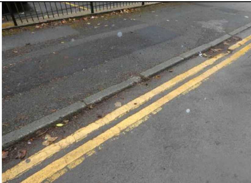
Photograph 22. Uneven and damaged kerb to George Street
