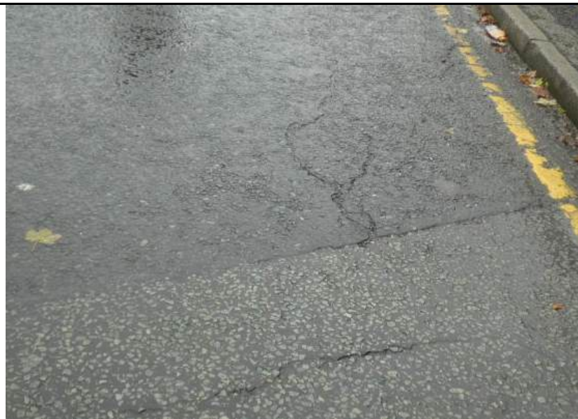
Photograph 82. Localised cracking to road surfacing.
