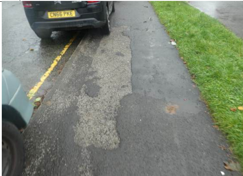
Photograph 68. Erosion to footpath
