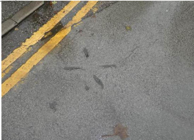
Photograph 28. Localised indentations to road surfacing
