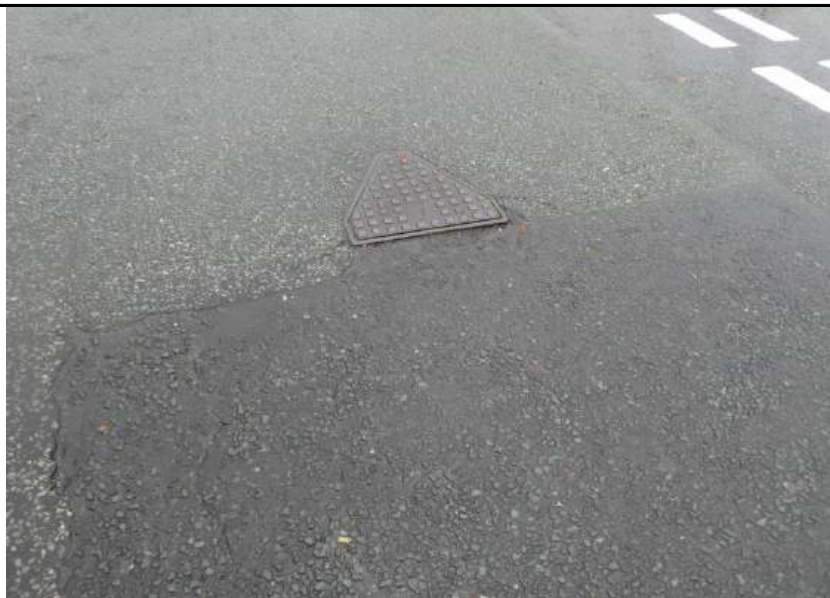
Photograph 90. Localised erosion to surfacing.
