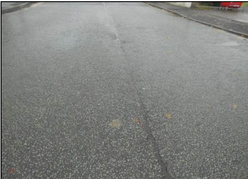
Photograph 81.Exposed joint to centre of roadway
