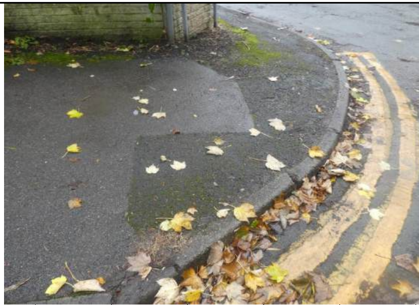
Photograph 14. Localised damage and settlement to the concrete kerbs
