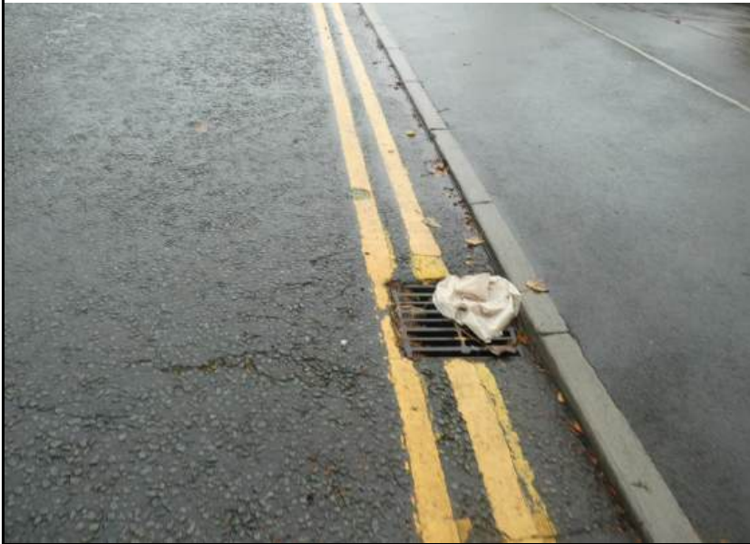
Photograph 43. Localised erosion to surfacing.
