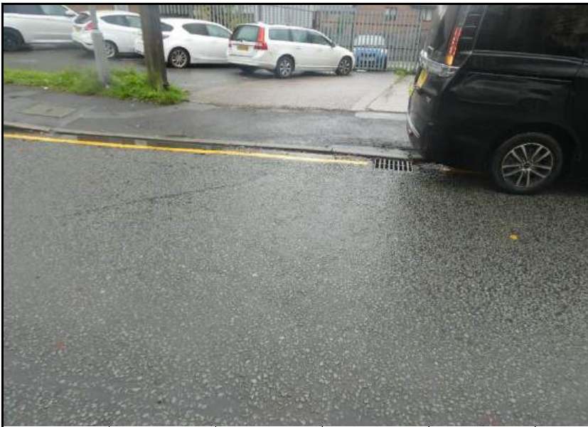
Photograph 61. Minor erosion to surfacing
