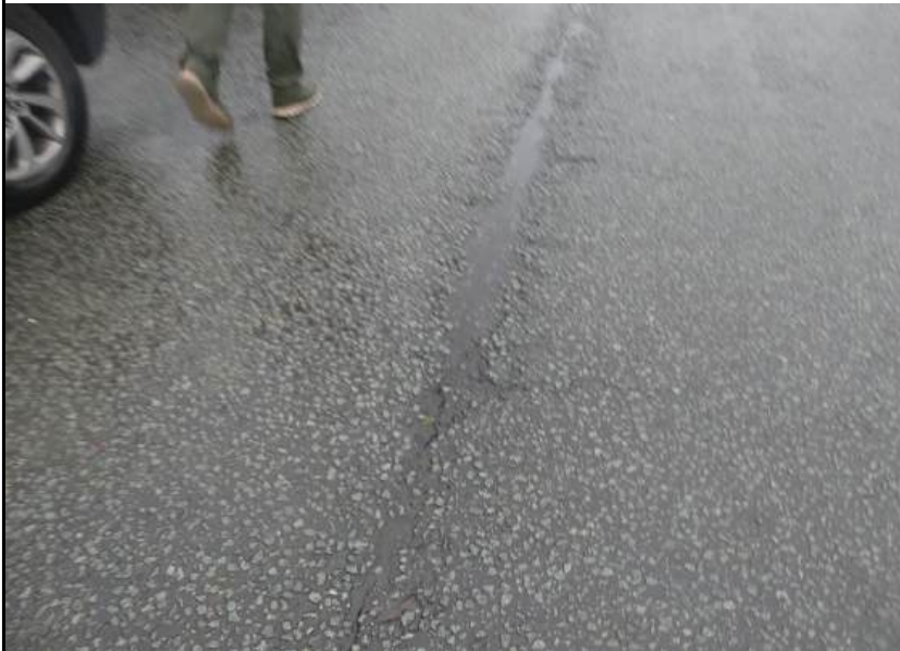
Photograph 59. Erosion to central section of roadway
