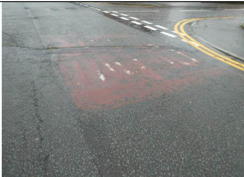
Photograph 46. Cracking to surfacing to centre of roadway.
