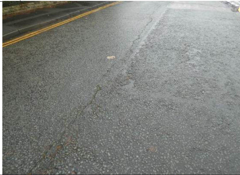
Photograph 44. Cracking to surfacing to centre of roadway.
