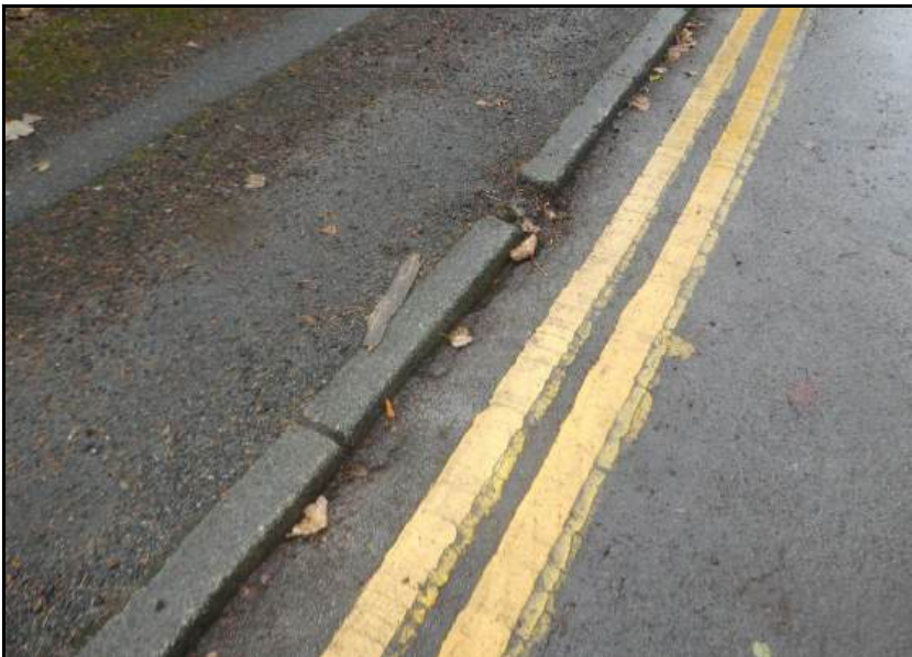
Photograph 21. Uneven and damaged kerb to George Street
