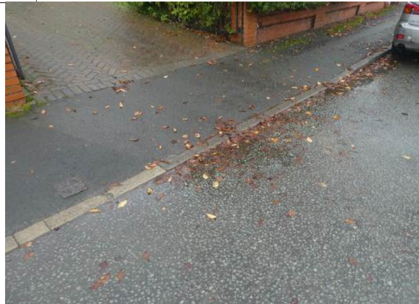
Photograph 60. Localised damage to kerbing
