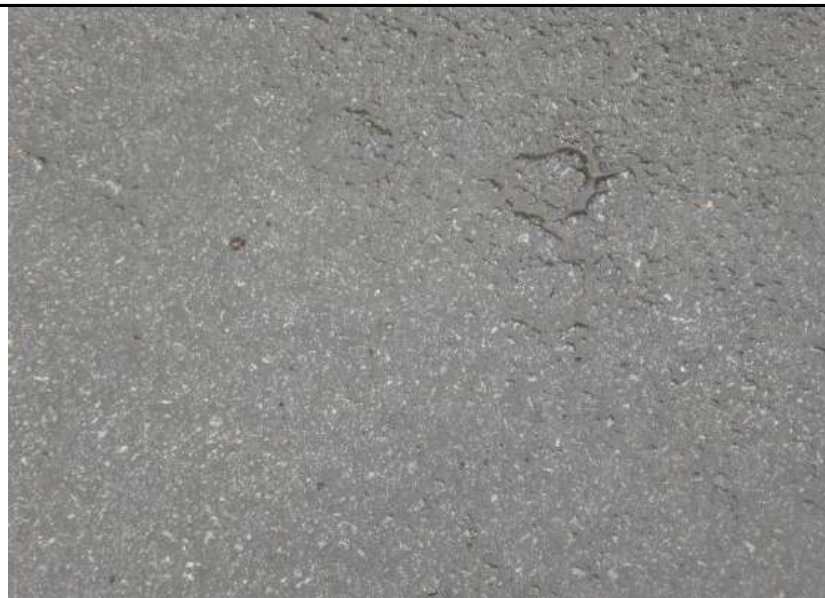
Photograph 10. Localised indentations to footpath areas
