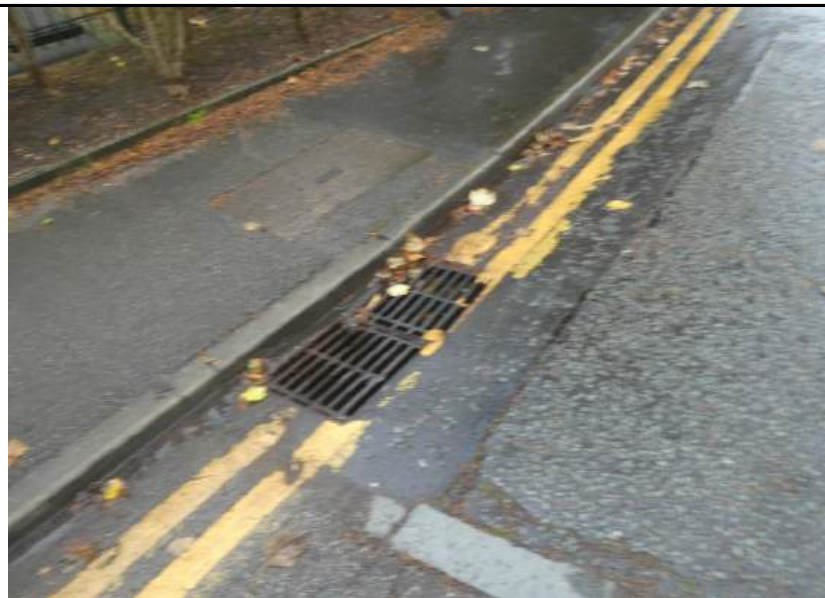
Photograph 34. Localised erosion to surfacing
