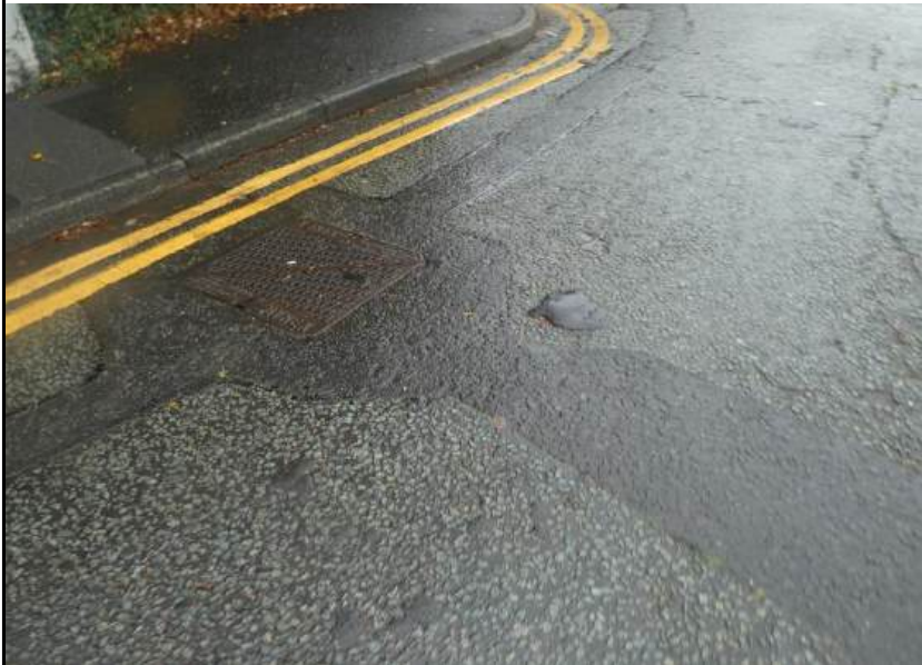
Photograph 47. Localised erosion to surfacing.
