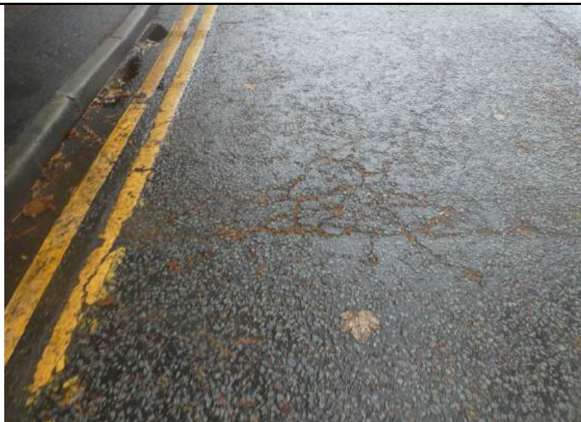
Photograph 38. Badly eroded and cracked surfacing
