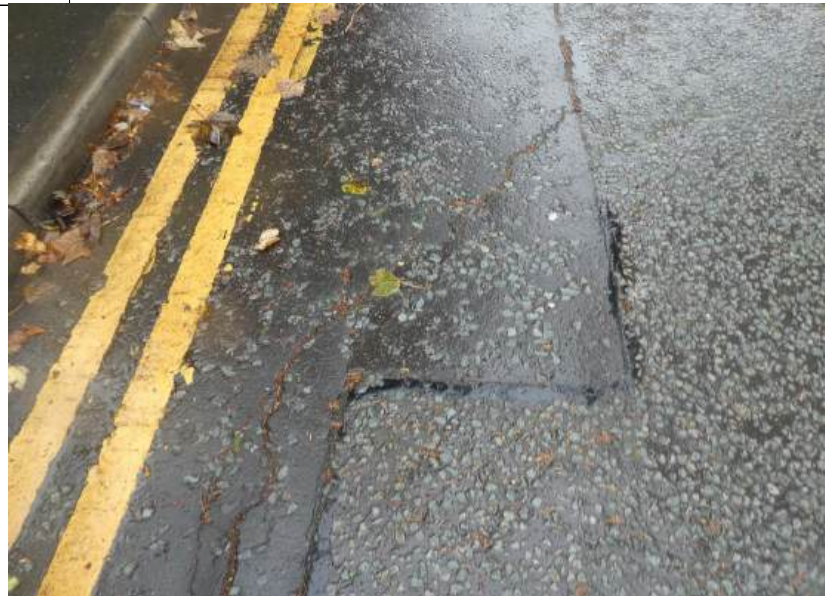
Photograph 36. Cracking to surfacing
