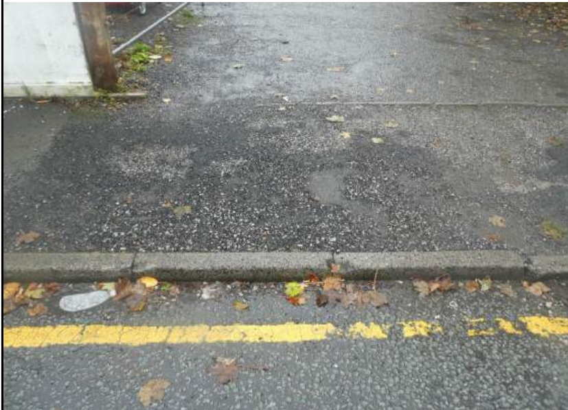
Photograph 83. Localised erosion to footpath
