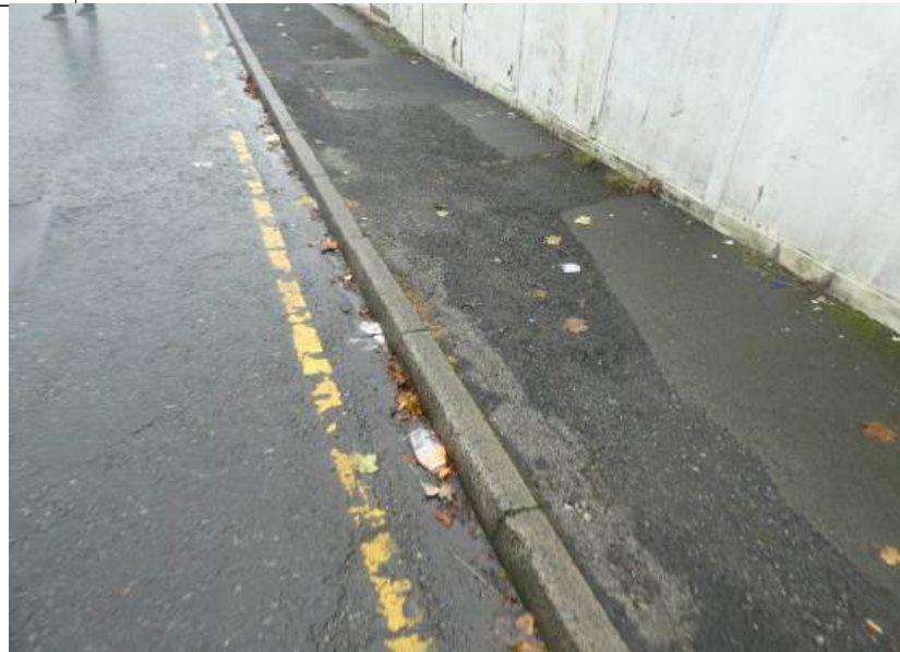
Photograph 84. Localised erosion to footpath.
