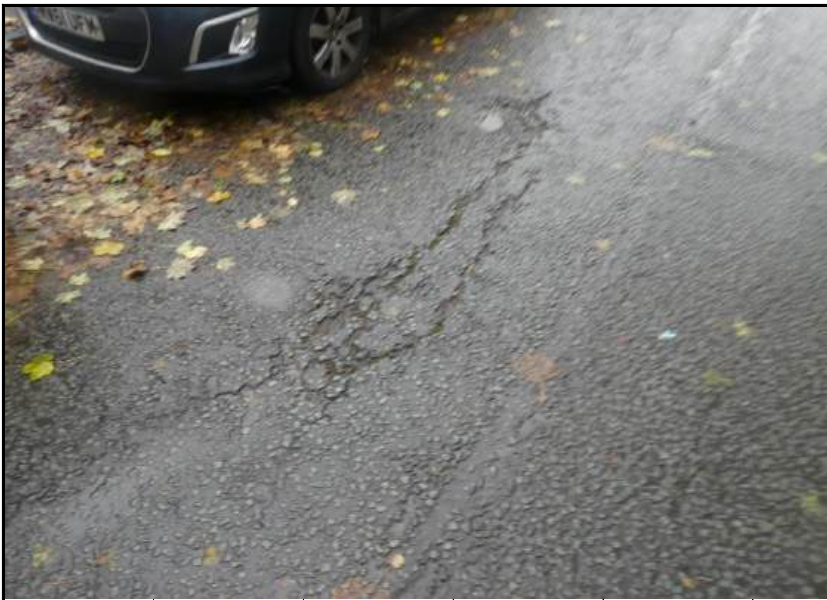
Photograph 77. Localised cracking to surfacing.
