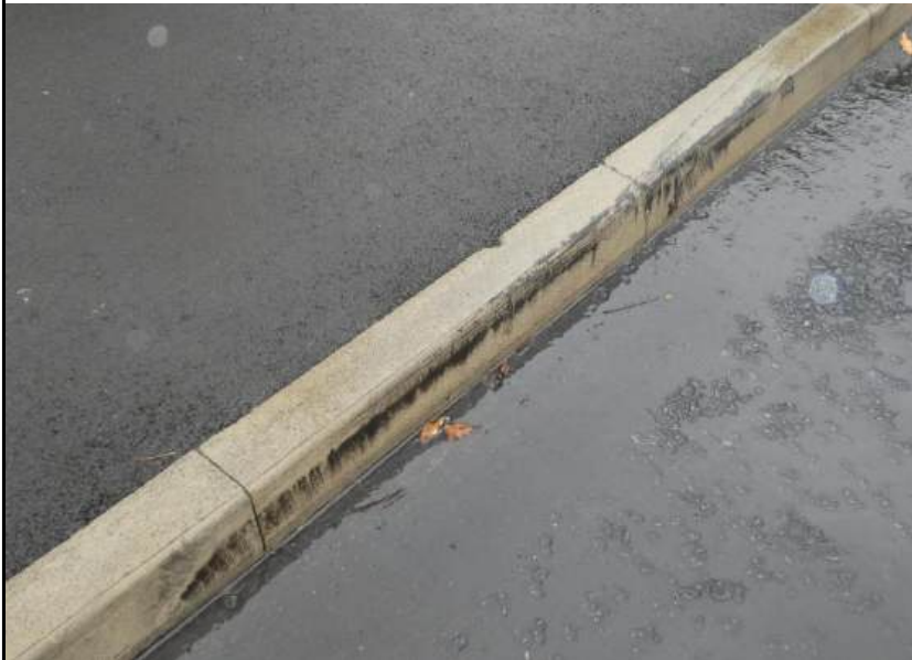
Photograph 7. Staining to the kerbing
