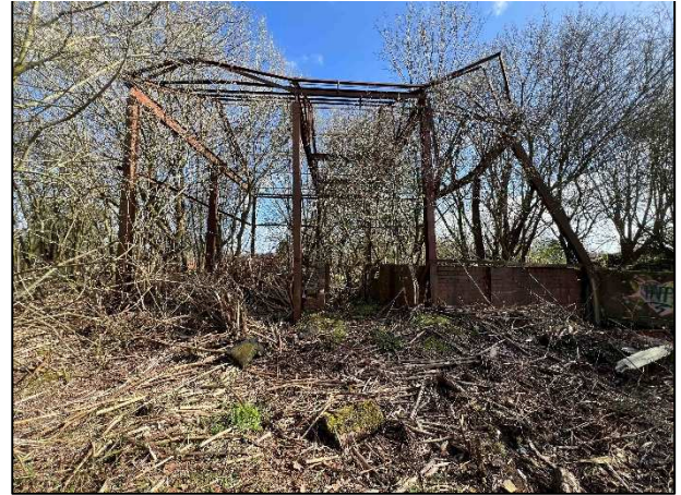
Photograph 6: Showing the dilapidated steel framed structure and large low level concrete structure
