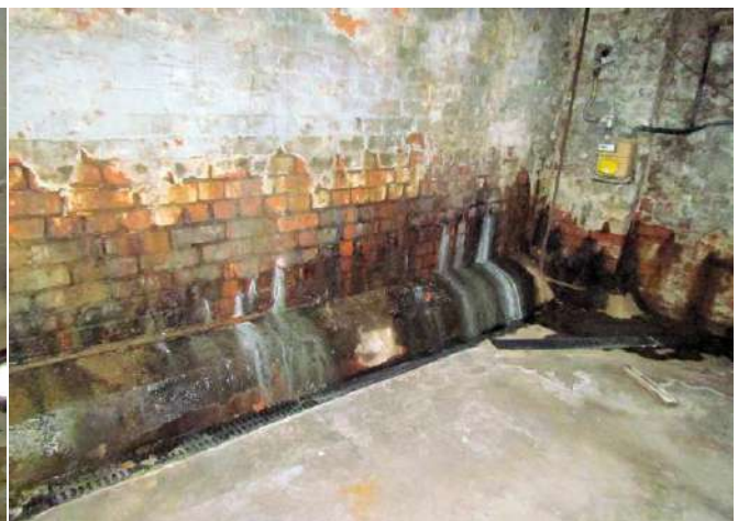
Flooding in Basement
