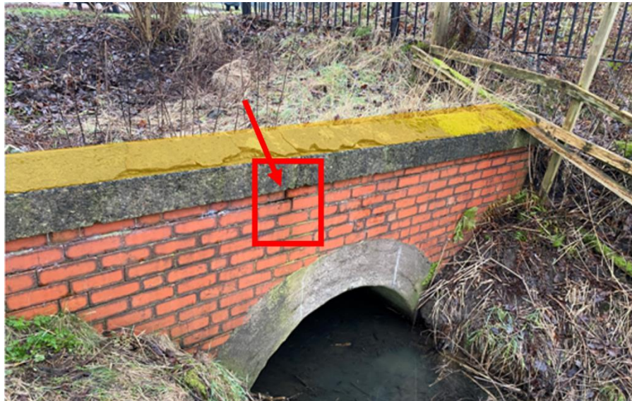
Photo. 1 Engineers Photo showing void in mortar (Indicated :taken prior to high rainfall event)
