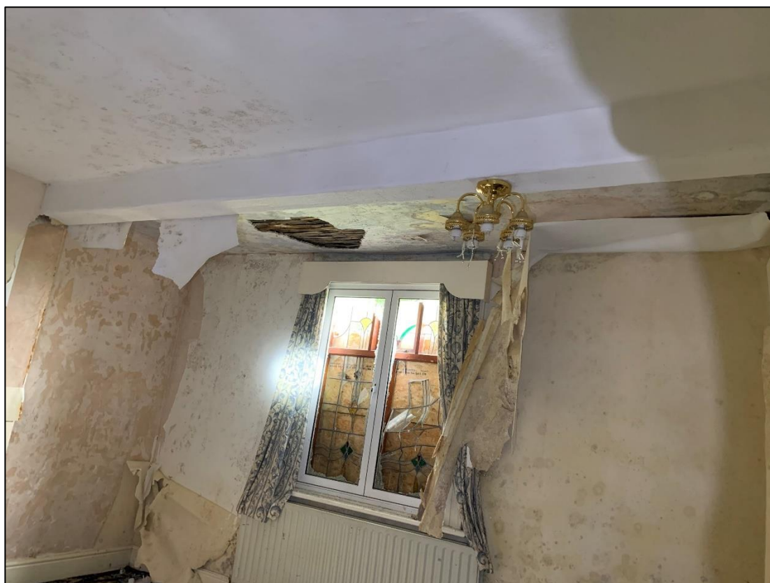
Plate 4 – Internal character of the building depicting water damage
