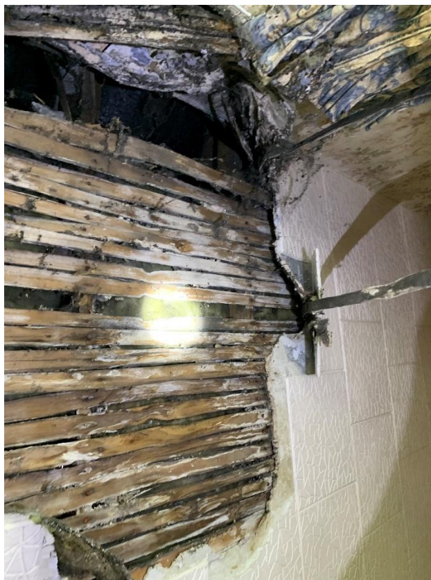
Plate 5 – Water damage tot first floor ceiling
