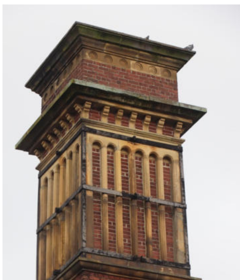
03 View of the cornice and decorative stonework at high level. Note unsightly staining and corrosion of metal strapping.
