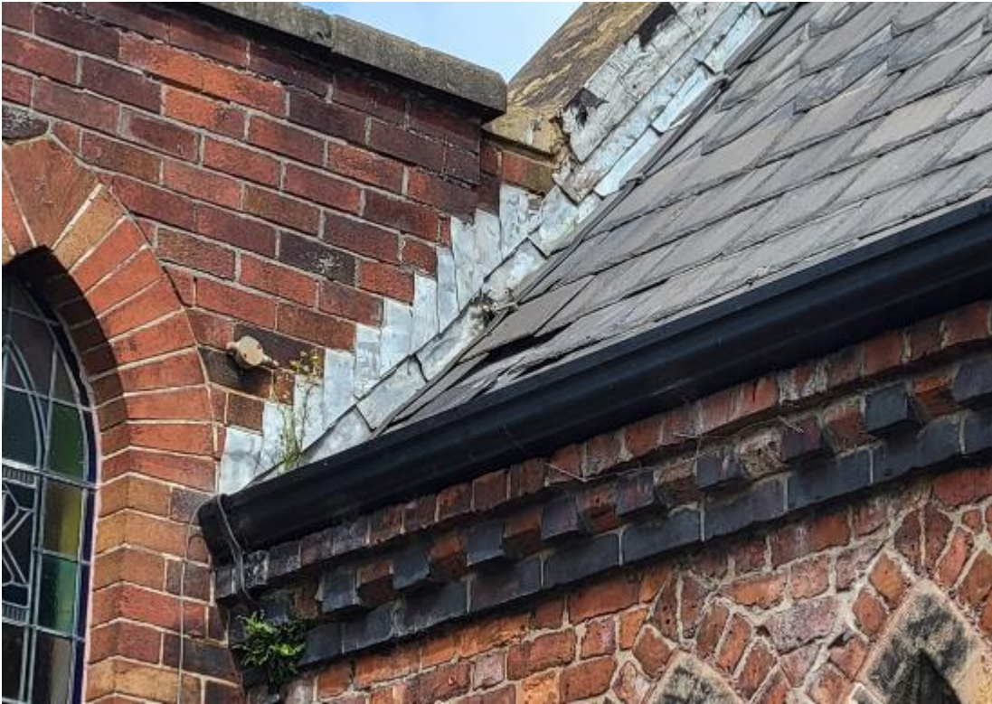
Plate B.9 Lifted slate roof tile on B2 located on the southern aspect, facing the garden courtyard
