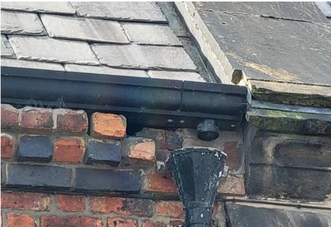
Plate B.8 Missing mortar on B2, located on the northern aspect facing Badger Street
