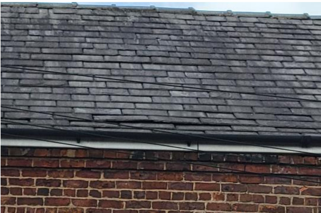
Plate B.6 Gaps underneath slate roof tiles on B3, facing the site boundary
