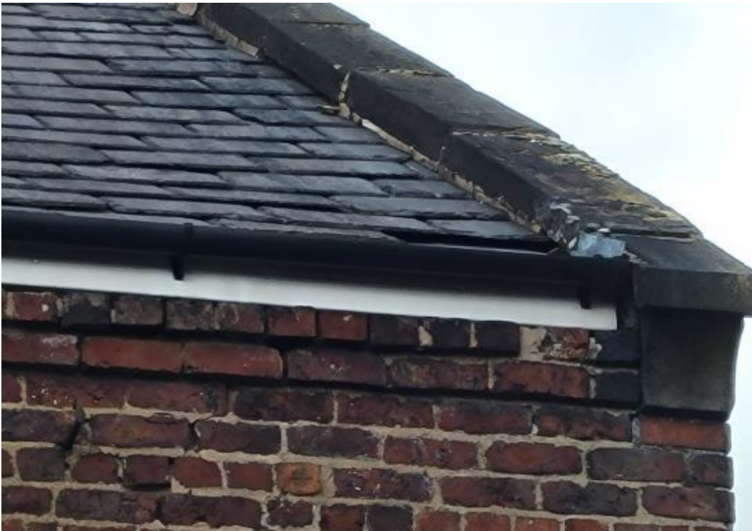
Plate B.5 Gaps underneath slate roof tiles on B3, facing the site boundary
