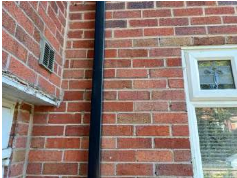
Photo 3: Stepped cracks in the brickwork of the existing building, potentially due to with shrink swell issues associated with nearby recently removed trees.
