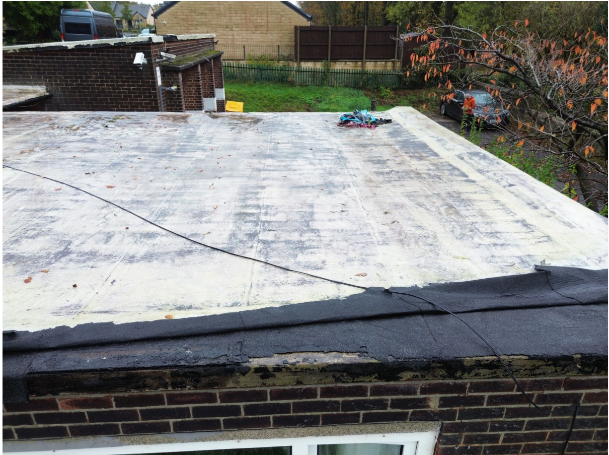
3 – There are small areas of damaged roofing felt but no viable gaps between materials.
