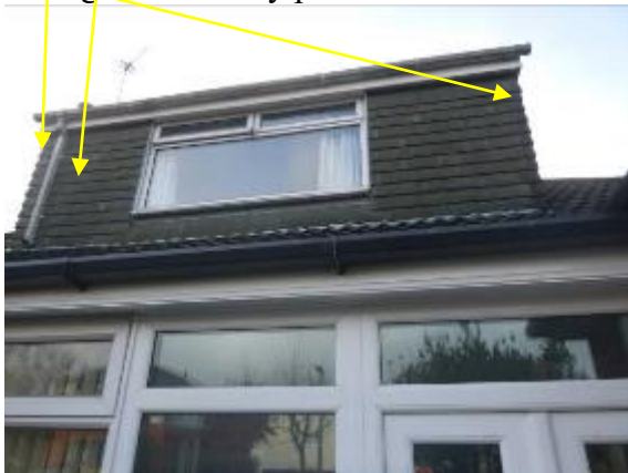
P3 Gaps at hanging tiles, front aspect
