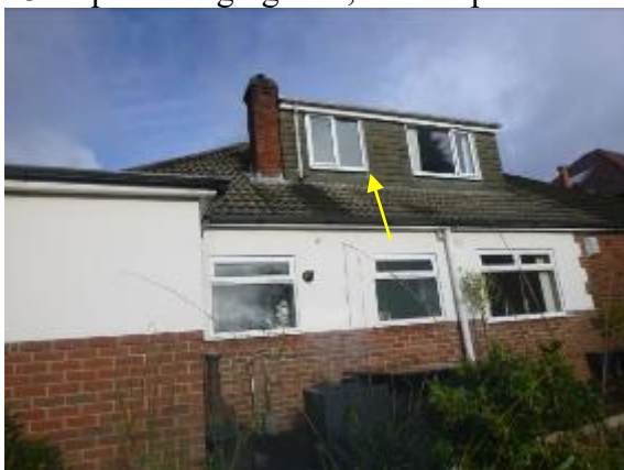
P5 Gaps at hanging tiles, rear aspect
