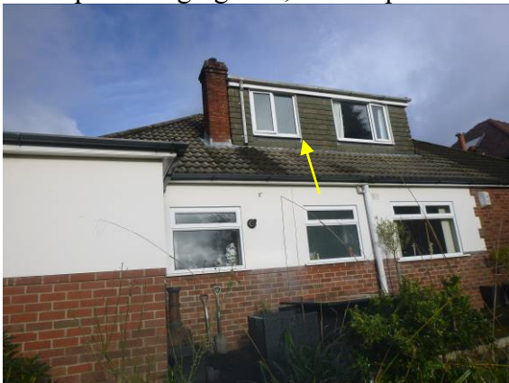
P5 Gaps at hanging tiles, rear aspect
