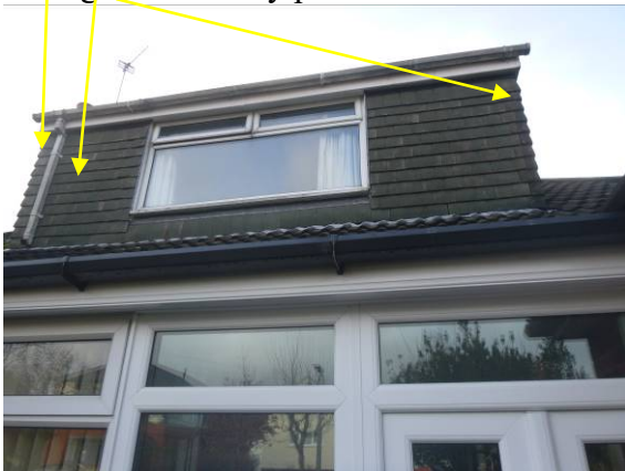
P3 Gaps at hanging tiles, front aspect
