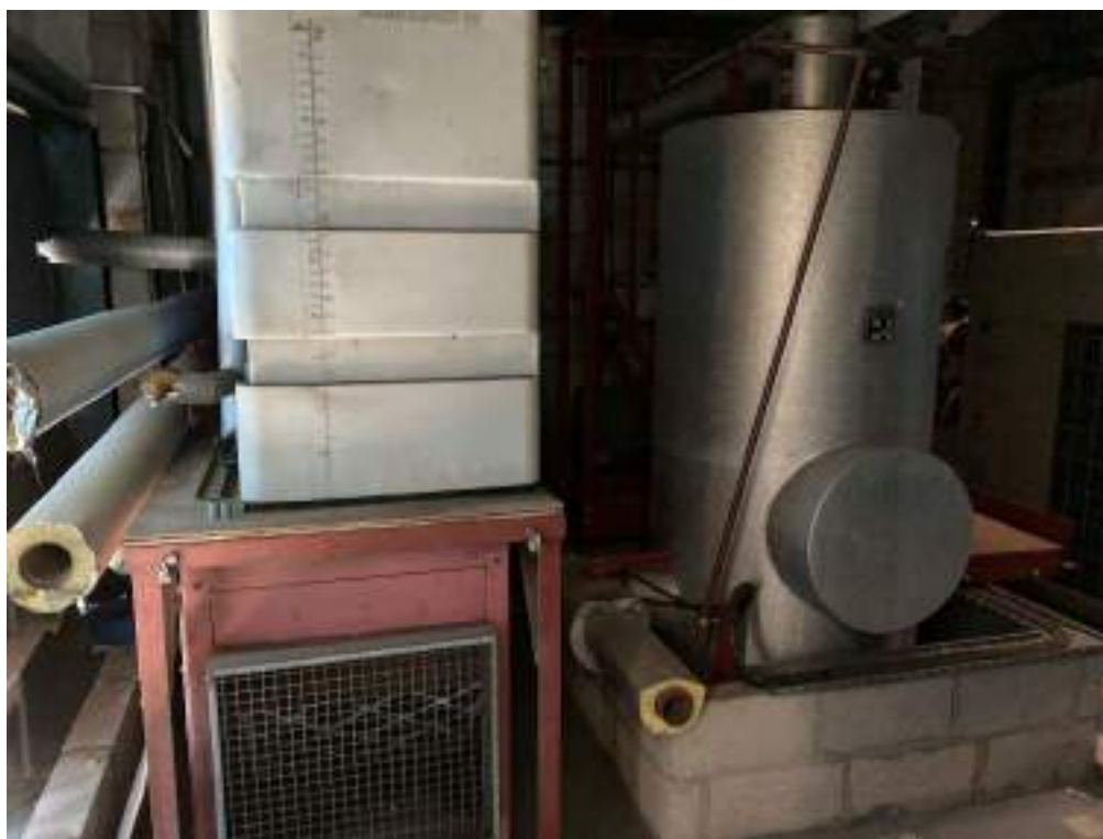
Photograph 16 – Southern plantroom (third floor)
