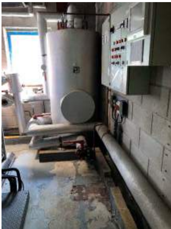
Photograph 16 - Northern plantroom (third floor)
