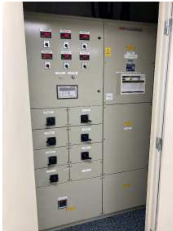
Photograph 14 - General switchboard (ground floor)
