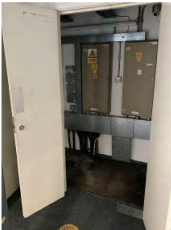
Photograph 15 - Switchboard (open space ground floor)
