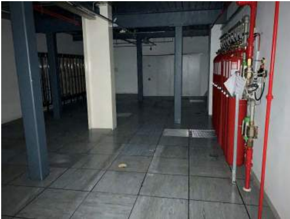
Photograph 13 - Inert Gas Fire Suppression System room (ground floor)
