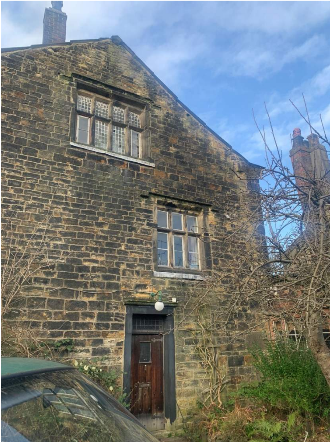
Figure 6 Image of eastern elevation showing bulge and cracking of stonework
