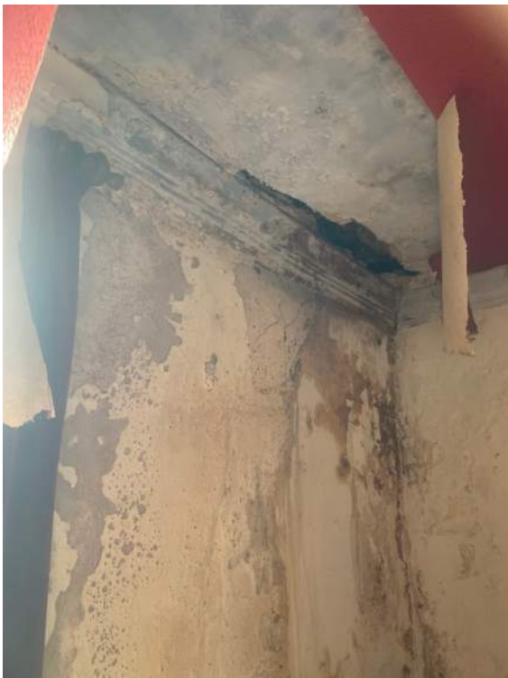
Figure 10 South western corner showing damage from water ingress
