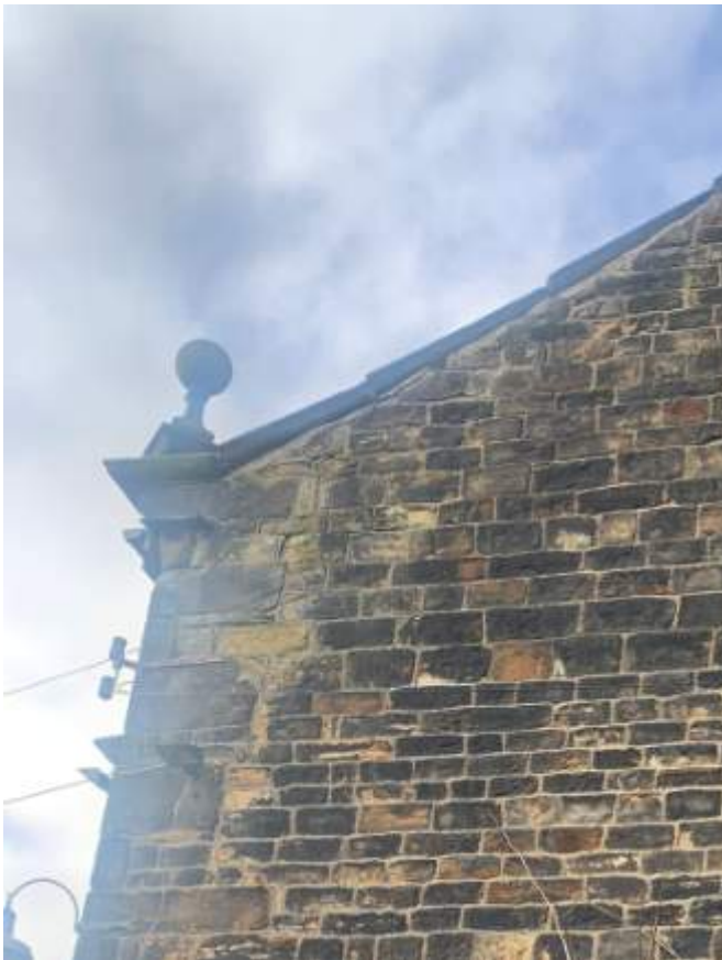
Figure 8 Cracking in stonework and movement of the kneeler
