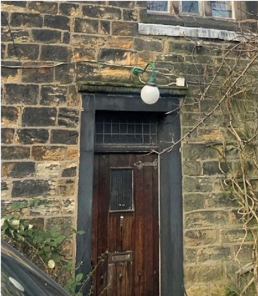
Figure 9 Cracked stone lintel and diagonal cracking in stonework above
