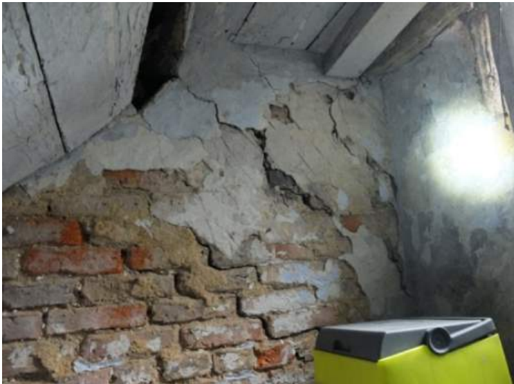
Figure 12 Cracking to basement cross walls running north south
