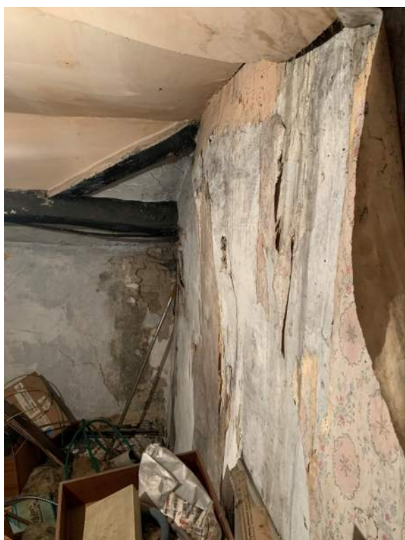
Figure 13 Significant internal bulge to north eastern bedroom
