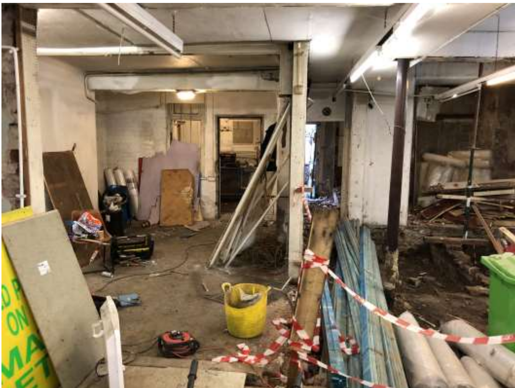
Image 10 – Internal view – significant repair/refurbishment required
