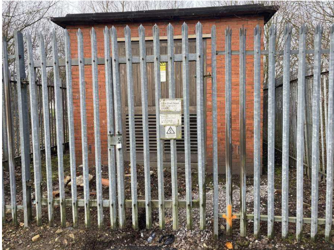
Plate 15 – Electrical substation in north west corner
