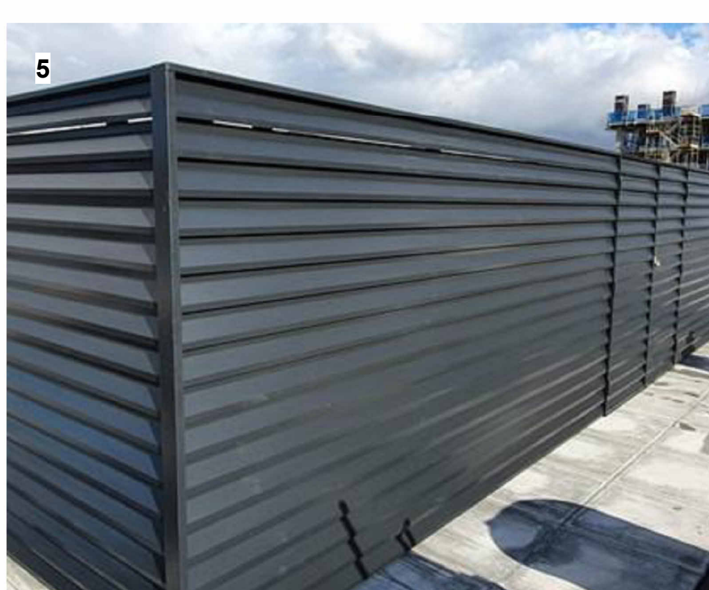
Louvre plant screen
