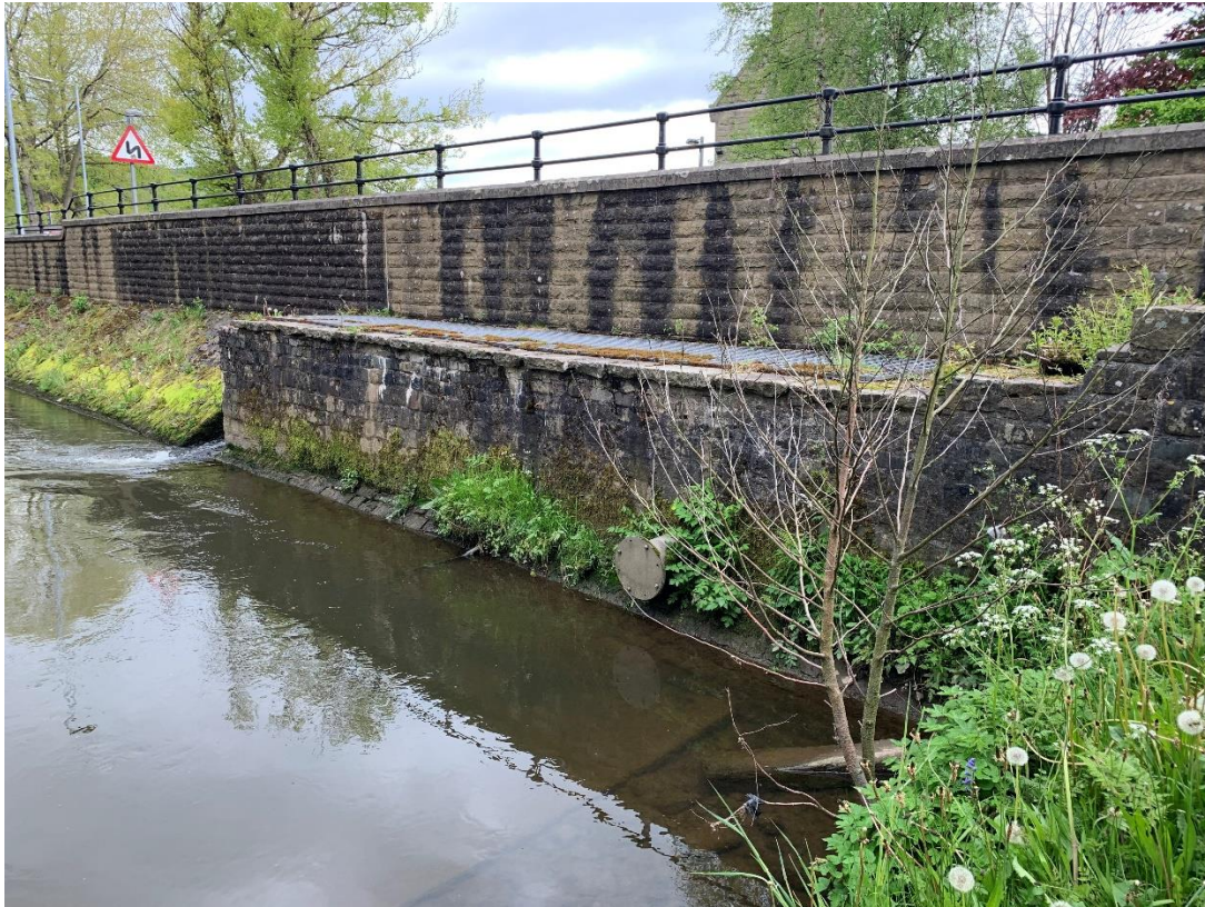
1 – Blanked off pipe inlet
