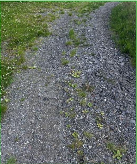
Showing the artificial unvegetated unsealed surface of the access.
