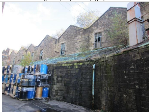
Photo 18: West elevation of Building 6; gaps present at broken window panes
