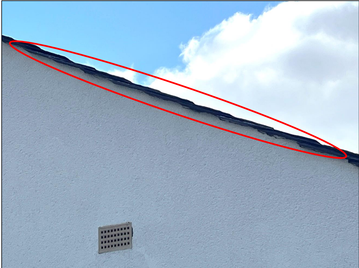
Plate 7 – Gaps at gable verges of B1
