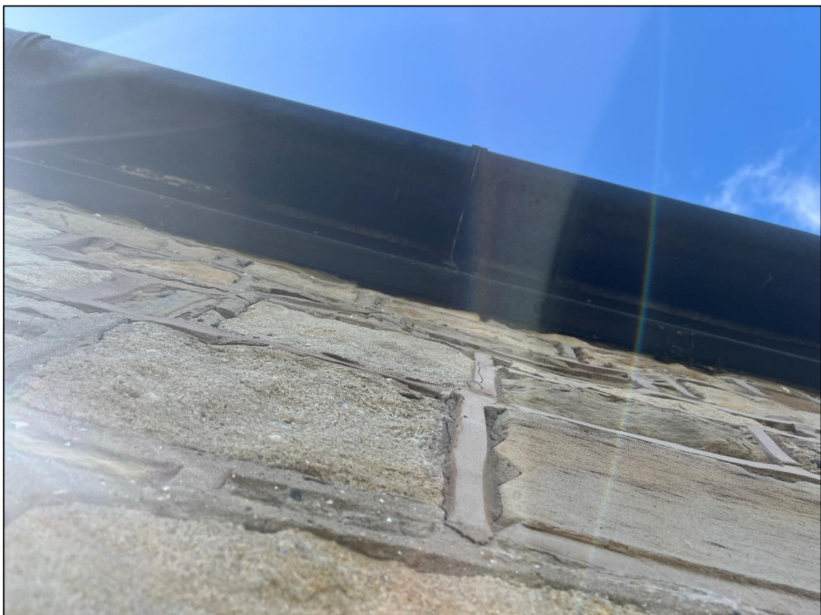
Plate 8 – Gaps beneath fascia of B1
