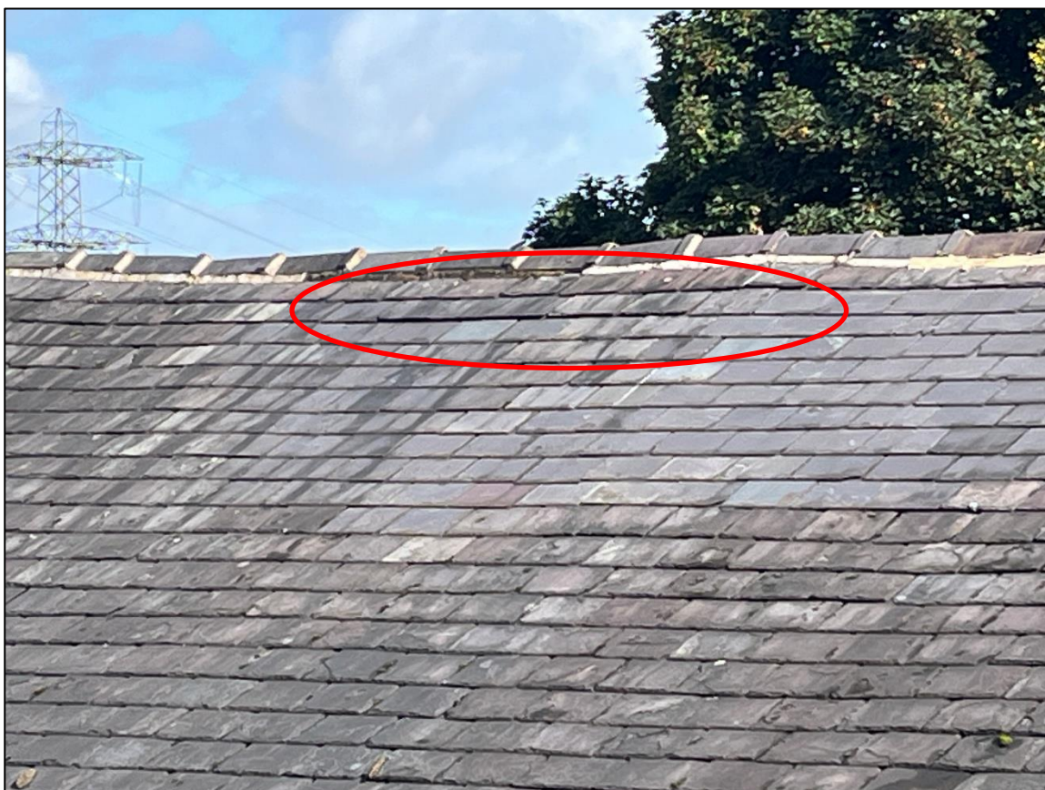
Plate 10 – Example of small number of lifted slates of B1
