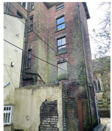
View from N Back Rock showing that refurbishment is required.
