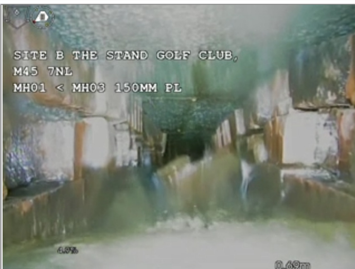
Survey abandoned - Remark: SA due to pipe size / shape change, unable to pass
