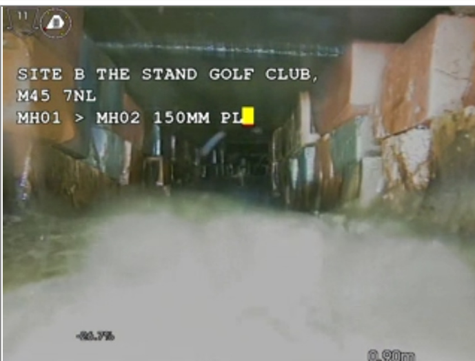
Survey abandoned - Remark: SA due to pipe size / shape change, unable to pass
