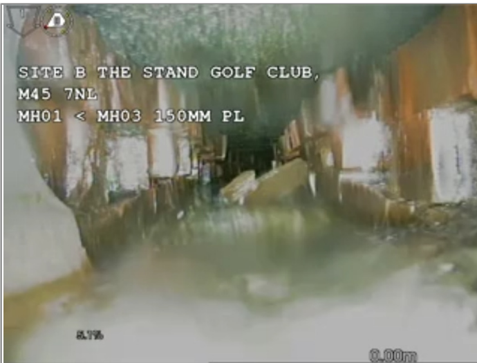
Start node type, Manhole, reference MH01
