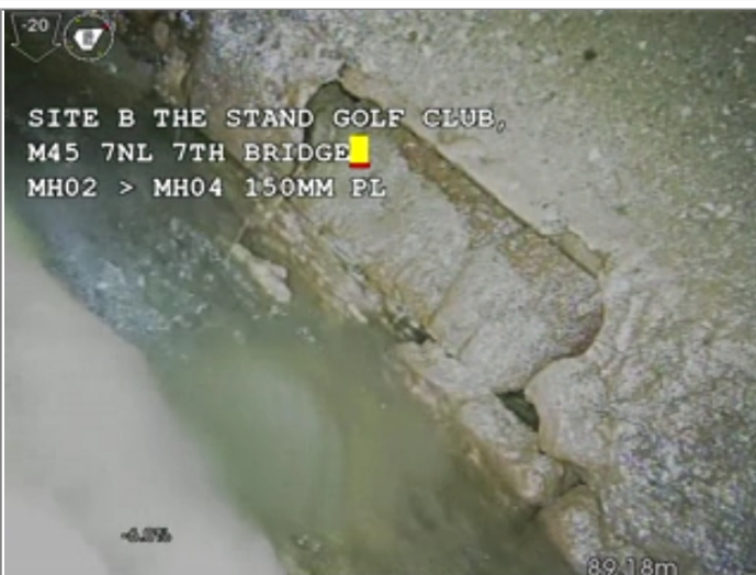
Finish node type, manhole, reference MH04
