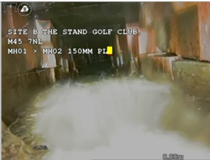
Start node type, Manhole, reference MH01
