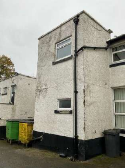
Fig.30 Structural failing [ Drees & Sommer]
