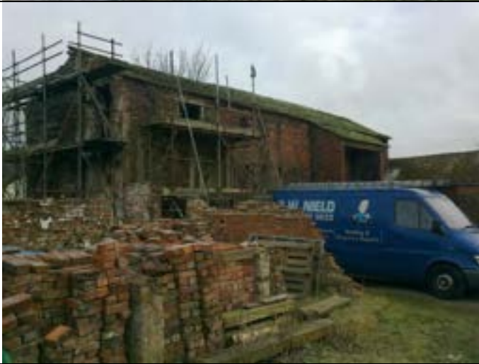
Photograph 5 (facing NW): Original farm building to the north west of the site. Bricks in the foreground are from a section of the building that blew down in the wind recently.
