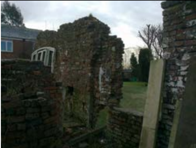
Photograph 6 (facing SE): Remains of the section of the building that blew down in the wind.
