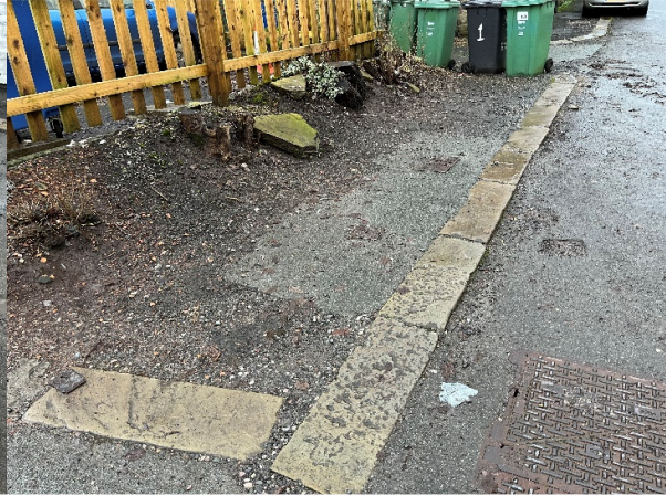
View 9 Spring Street left side pavement
