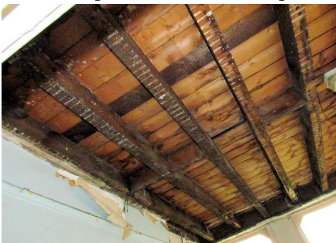
Ceiling Gone, 2 nd Floor
