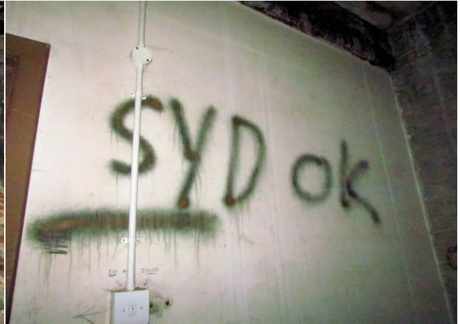
Evidence of Vandalism
