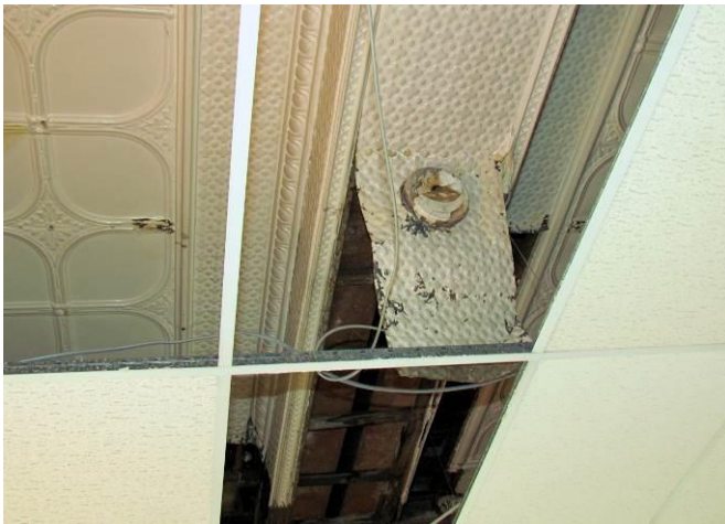
Damaged Pressed Steel Ceiling
