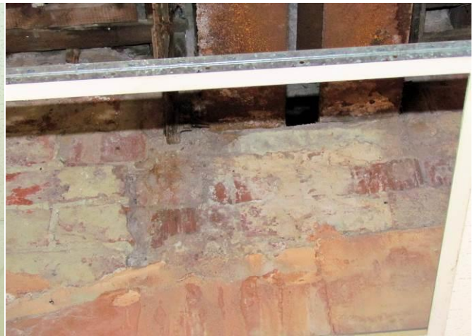
Rusting Structural Beam
