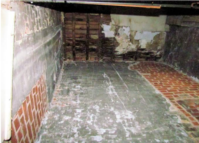
Ceiling Collapsed Above North Staircase
