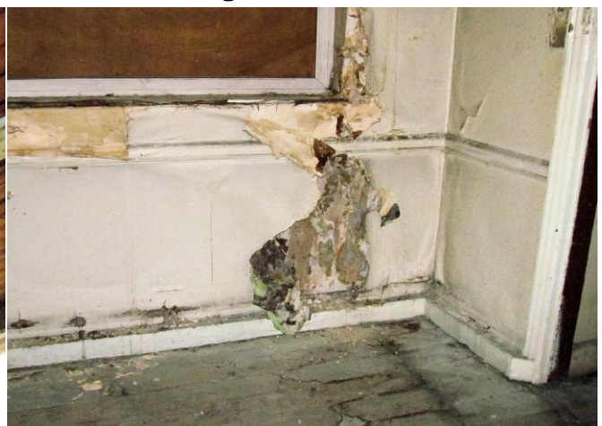
Damp in North Wall, West Side
