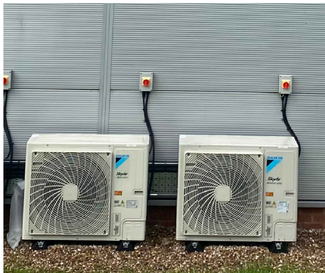
PHOTO OF TYPICAL LOW LEVEL FLOOR MOUNTED AIR SOURCE HEAT PUMPS NOT TO SCALE
