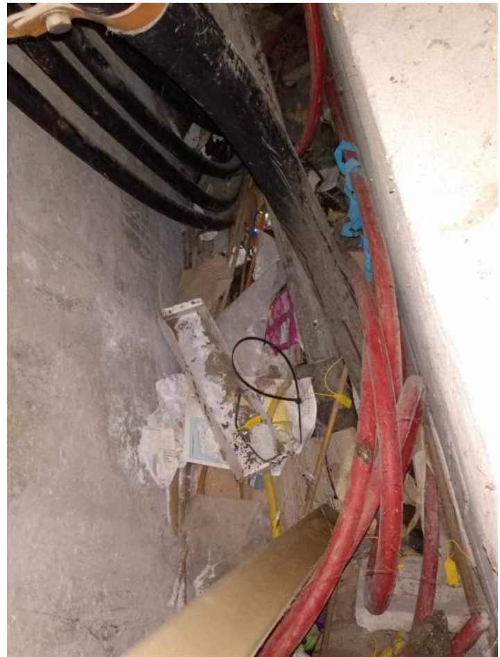
68) Electrical cables in pit in boiler house
