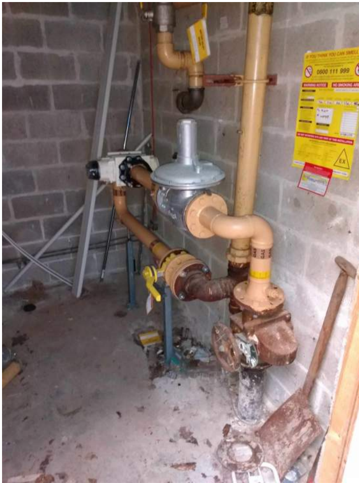
65) Boiler house interior
