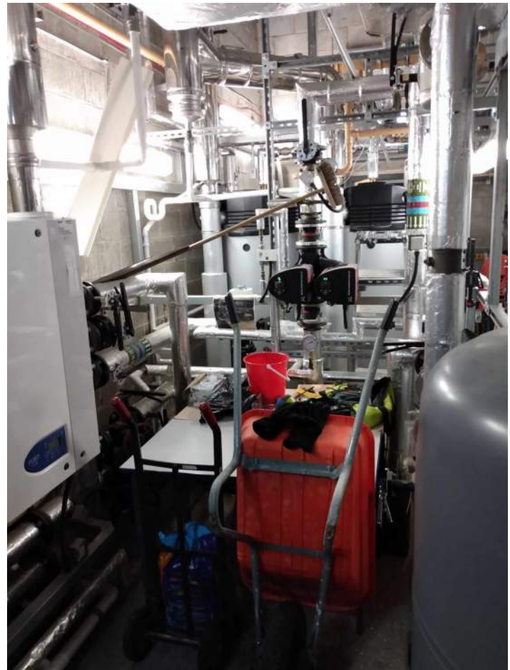
52) Plant Room (Boiler Room) of Spring Lane School
