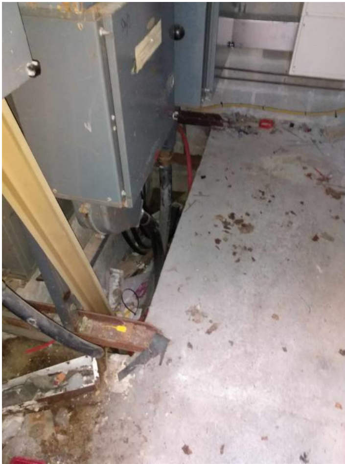
67) Boiler house interior
