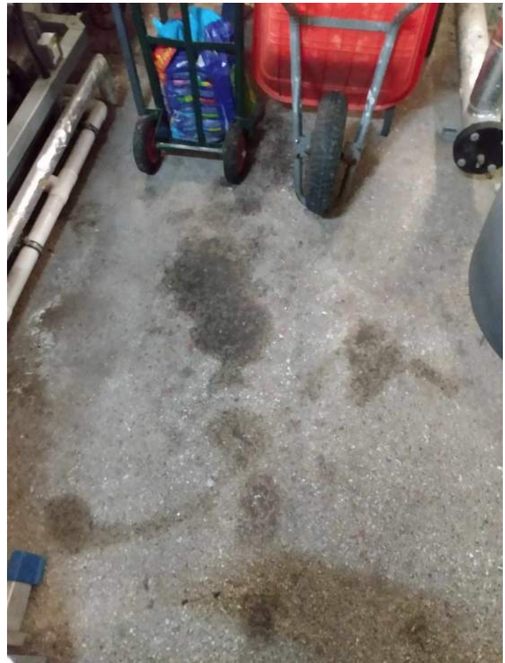
50) Possible oil stains on Plant Room floor
