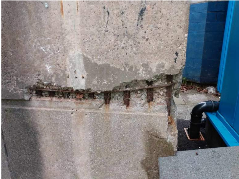
61) Corrosion to steel reinforcing bars and concrete of boiler house chimney
