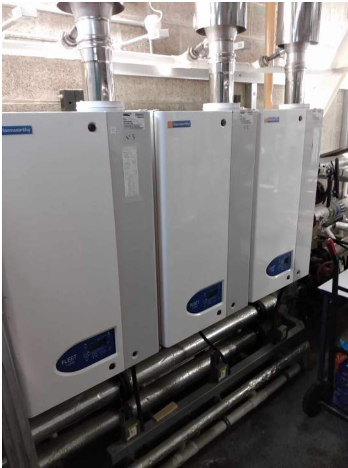
51) Plant Room (Boiler Room) of Spring Lane School
