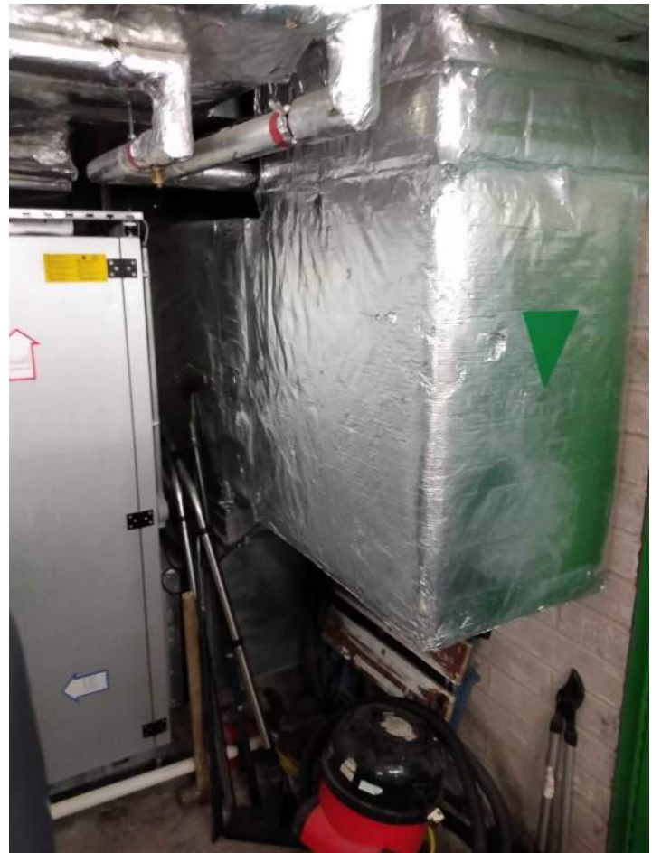
54) Plant Room (Boiler Room) of Spring Lane School
