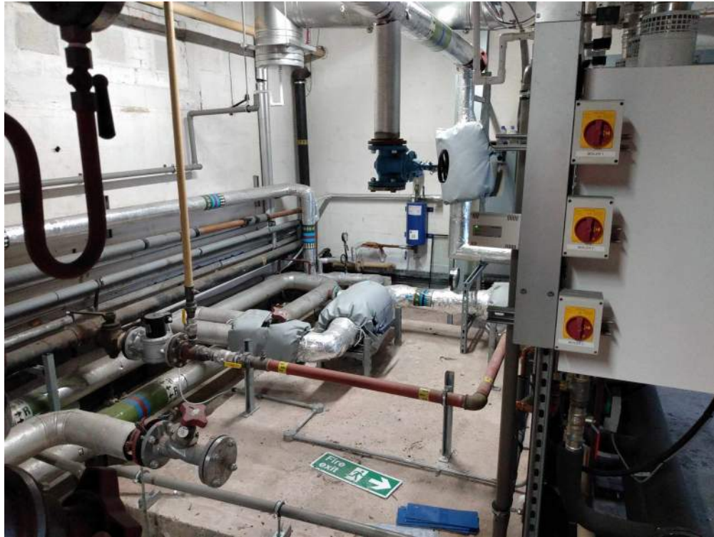
63) Boiler house interior
