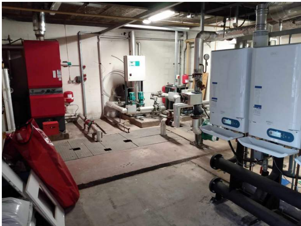
62) Boiler house interior
