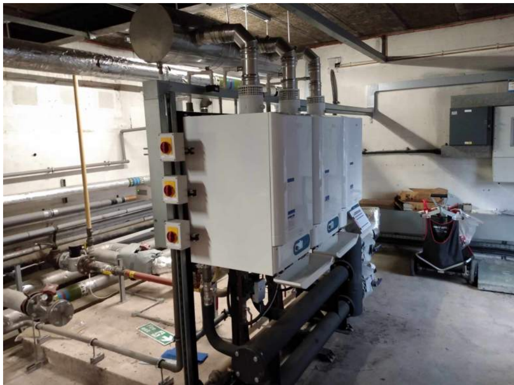
64) Boiler house interior
