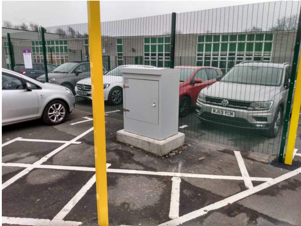
37) Electrical service box in car park on north side of Spring Lane School
