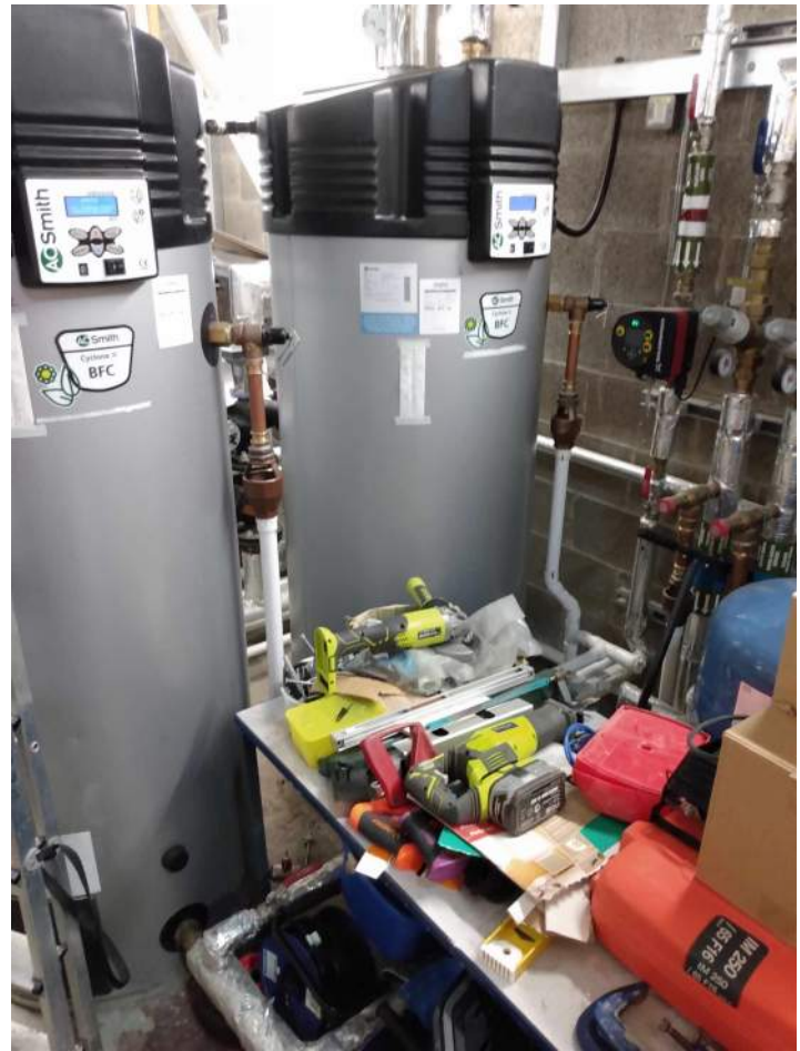
56) Plant Room (Boiler Room) of Spring Lane School
