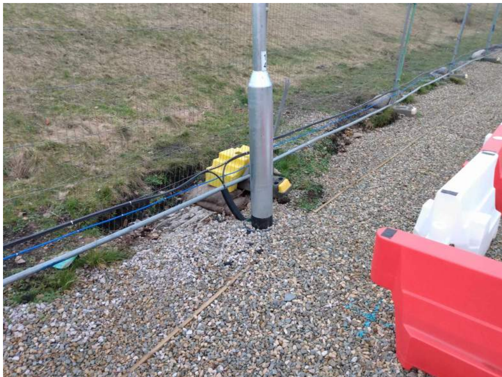
34) Electricity cables to lighting columns along west side of new gravel-surfaced car parking area
