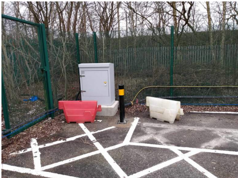
38) Electrical service box in northeast corner of car park north of Spring Lane School
