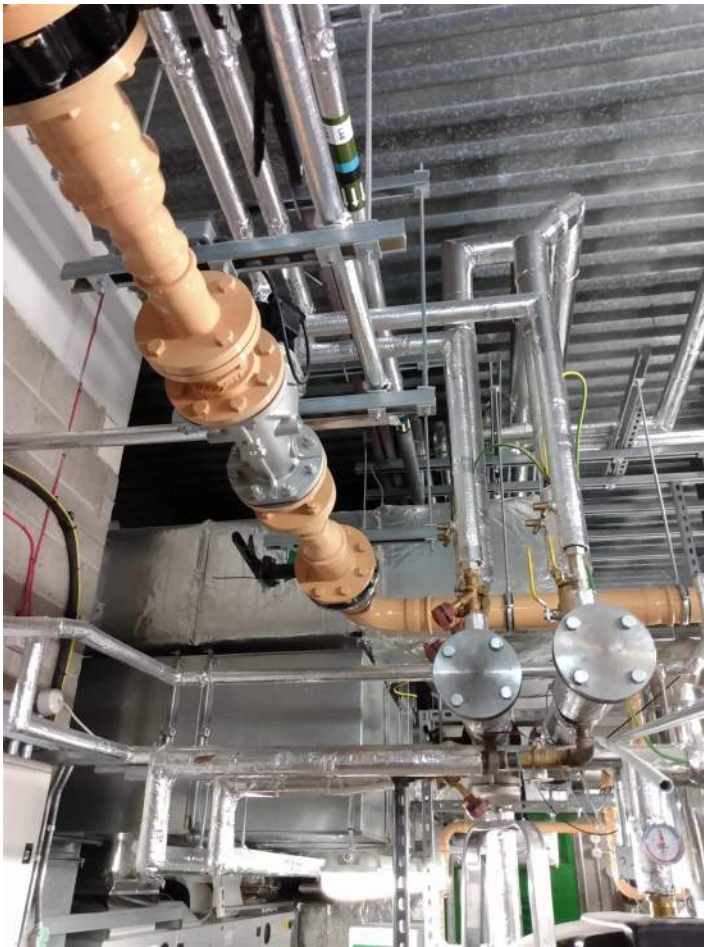
55) Plant Room (Boiler Room) of Spring Lane School
