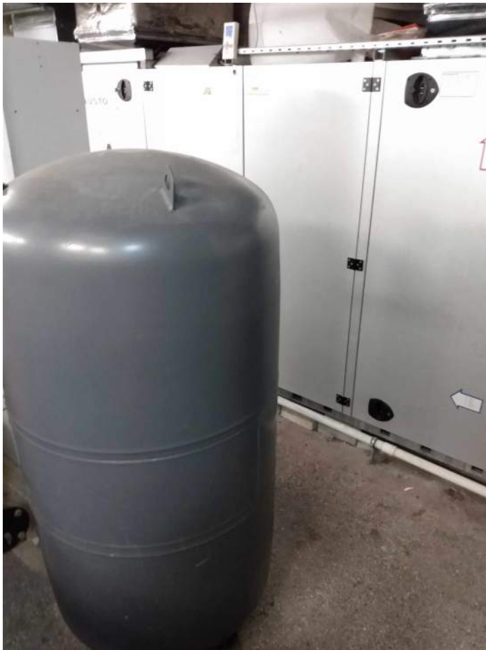
53) Plant Room (Boiler Room) of Spring Lane School
