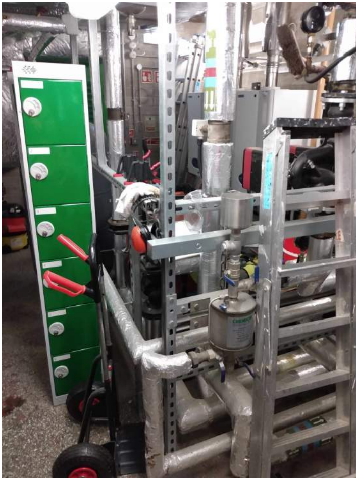
49) Plant Room (Boiler Room)
