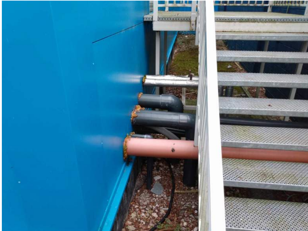
71) Pipework from blue swimming pool building passing under stairs to the filtration unit
