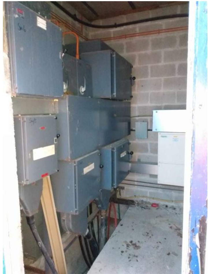
66) Boiler house interior
