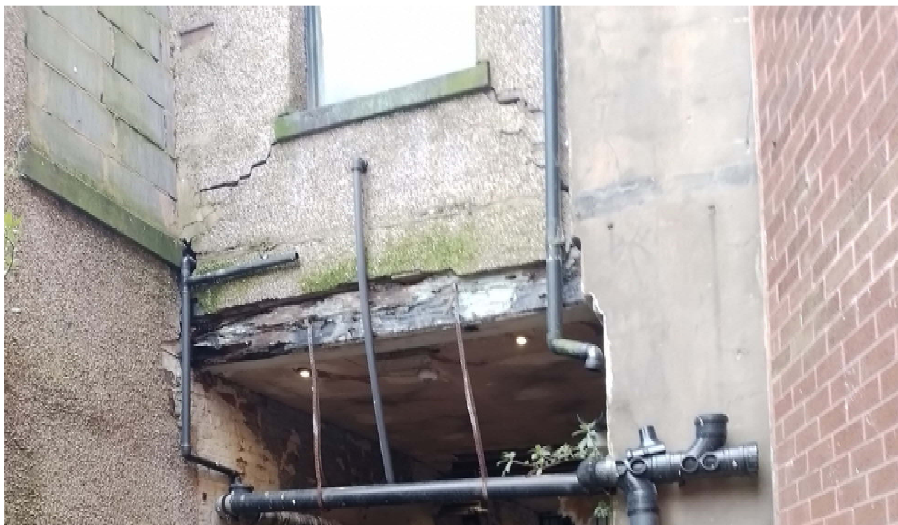
Photograph 6 - Subsidence damage on existing building in the south.
