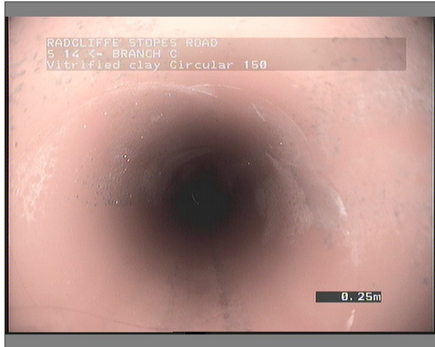
Photo: 7_7_28_A.JPG 0.25m, Crack, circumferential, from 12 to 12 o'clock
