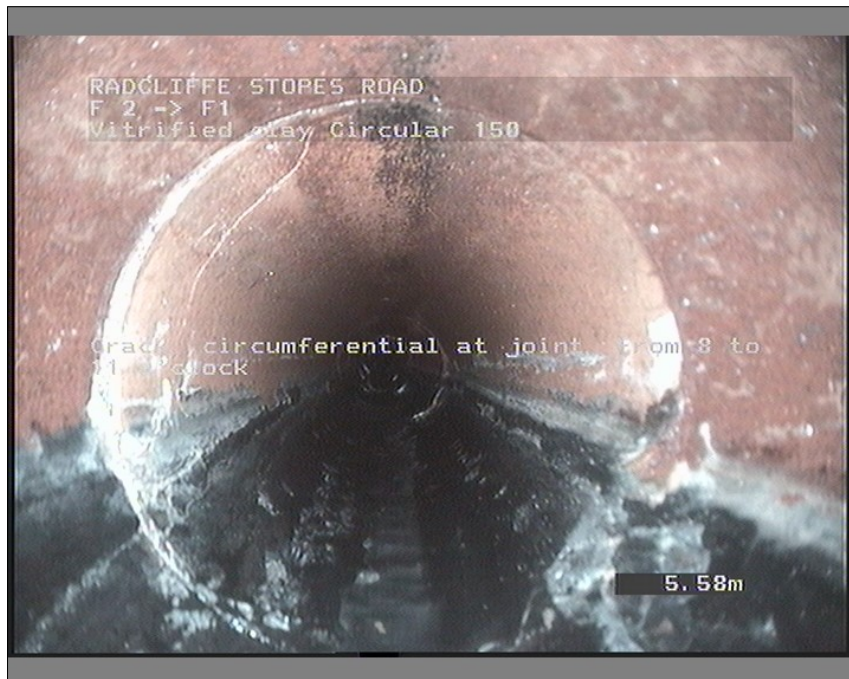
Photo: 15_15_86_A.JPG 5.58m, Crack, circumferential at joint, from 8 to 11 o'clock
