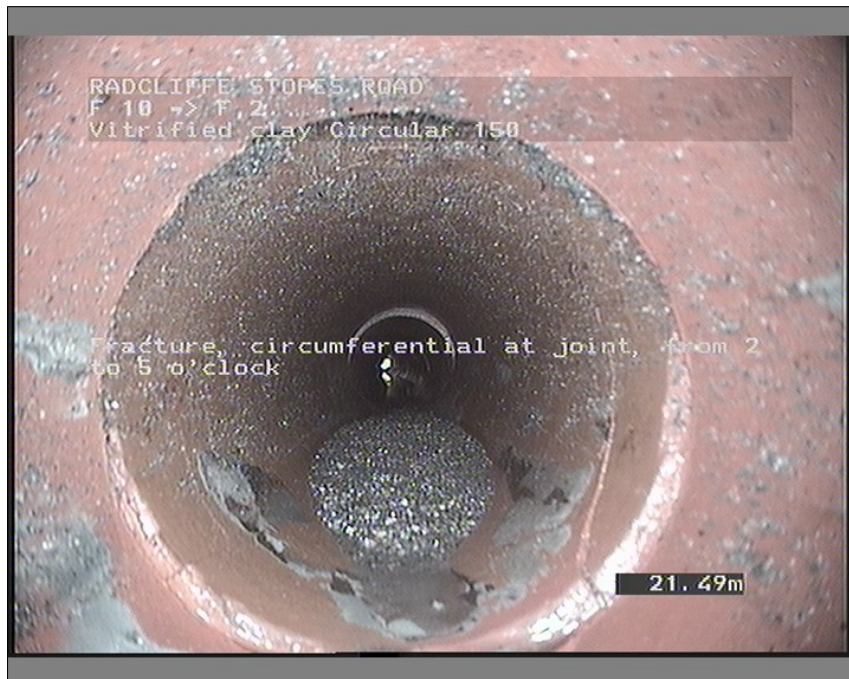
Photo: 12_12_69_A.JPG 21.49m, Fracture, circumferential at joint, from 2 to 5 o'clock
