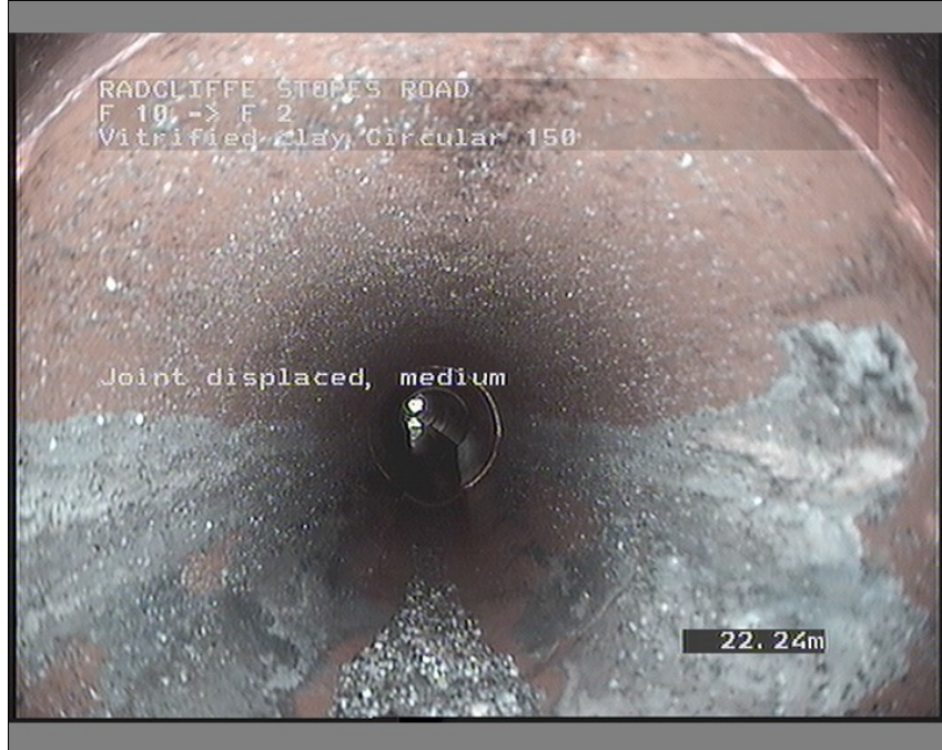
Photo: 12_12_70_A.JPG 22.24m, Joint displaced, medium
