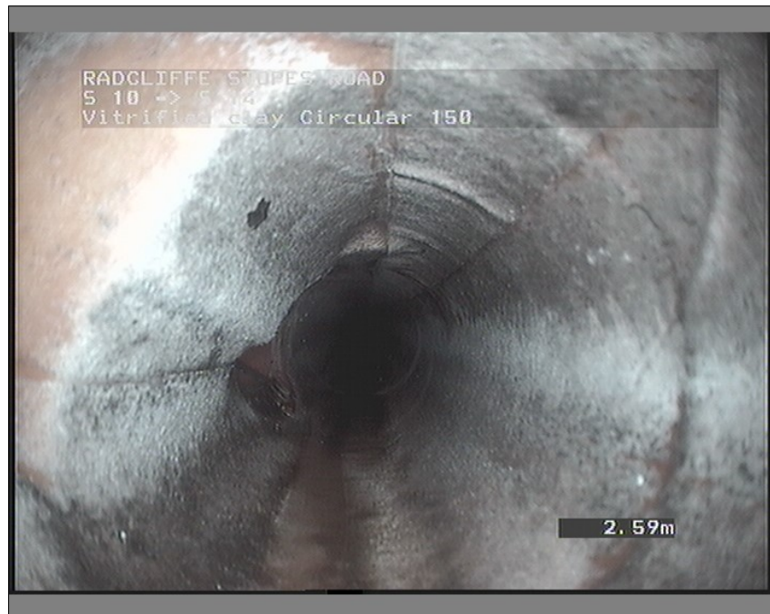
Photo: 8_8_34_A.JPG 2.59m, Deformed sewer/drain, 10%
