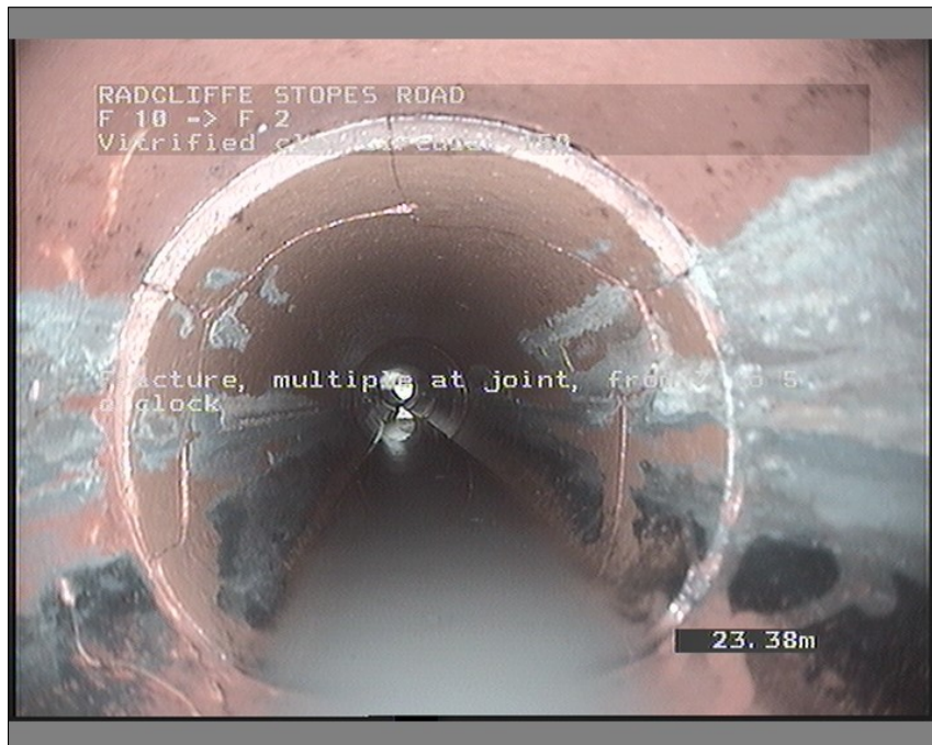
Photo: 12_12_71_A.JPG 23.38m, Fracture, multiple at joint, from 7 to 5 o'clock
