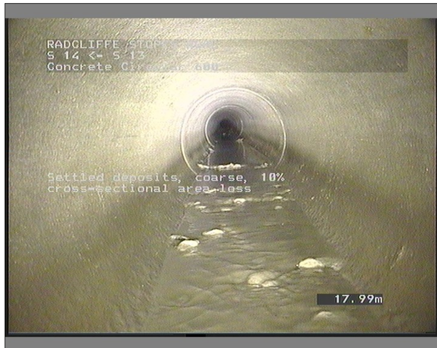
Photo: 1_1_4_A.JPG 17.99m, Settled deposits, coarse, 10% cross-sectional area loss
