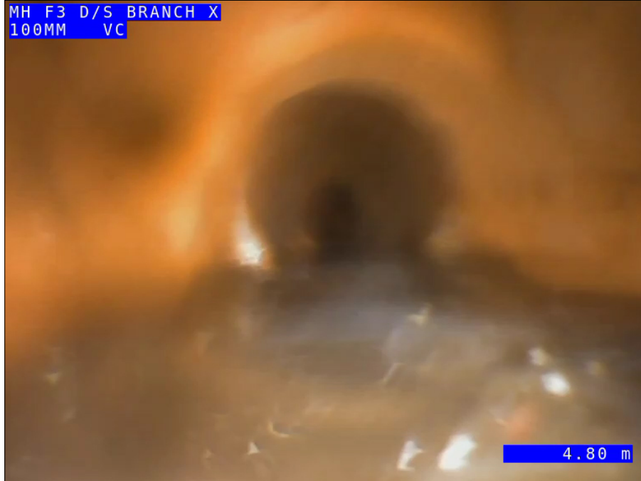
Photo: 17_17_103_A.jpg 4.88m, Junction, at 11 o'clock, diameter 100mm
