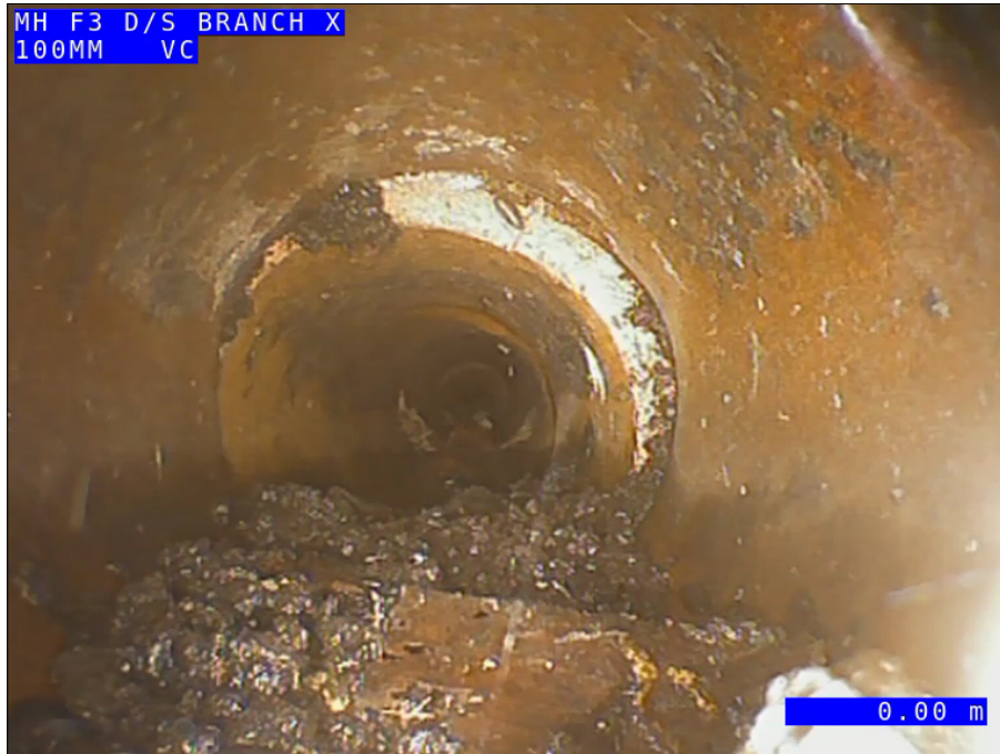
Photo: 16_16_97_A.jpg 0m, Settled deposits, coarse, 10% cross-sectional area loss
