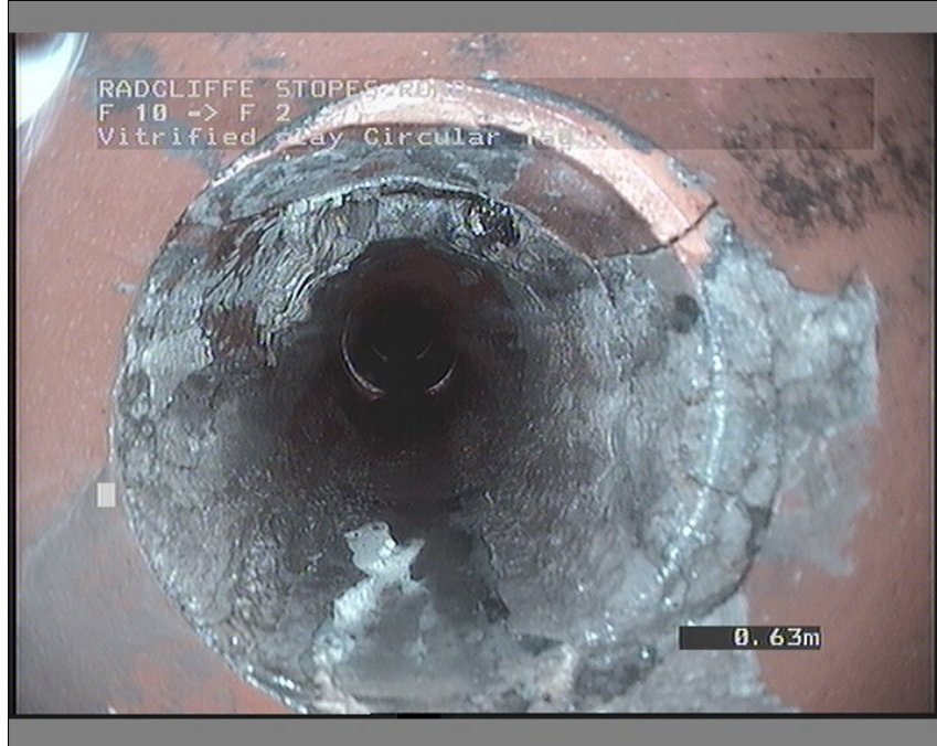
Photo: 12_12_62_A.JPG 0.63m, Fracture, circumferential at joint, from 10 to 4 o'clock
