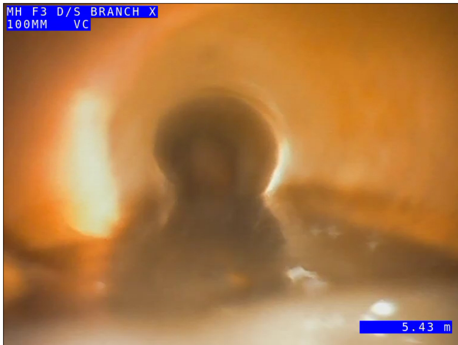
Photo: 17_17_104_A.jpg 5.43m, Junction, at 11 o'clock, diameter 100mm
