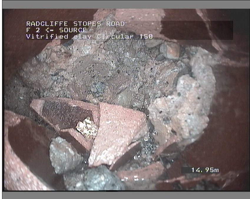
Photo: 14_14_83_A.JPG 14.95m, Collapsed drain/sewer
