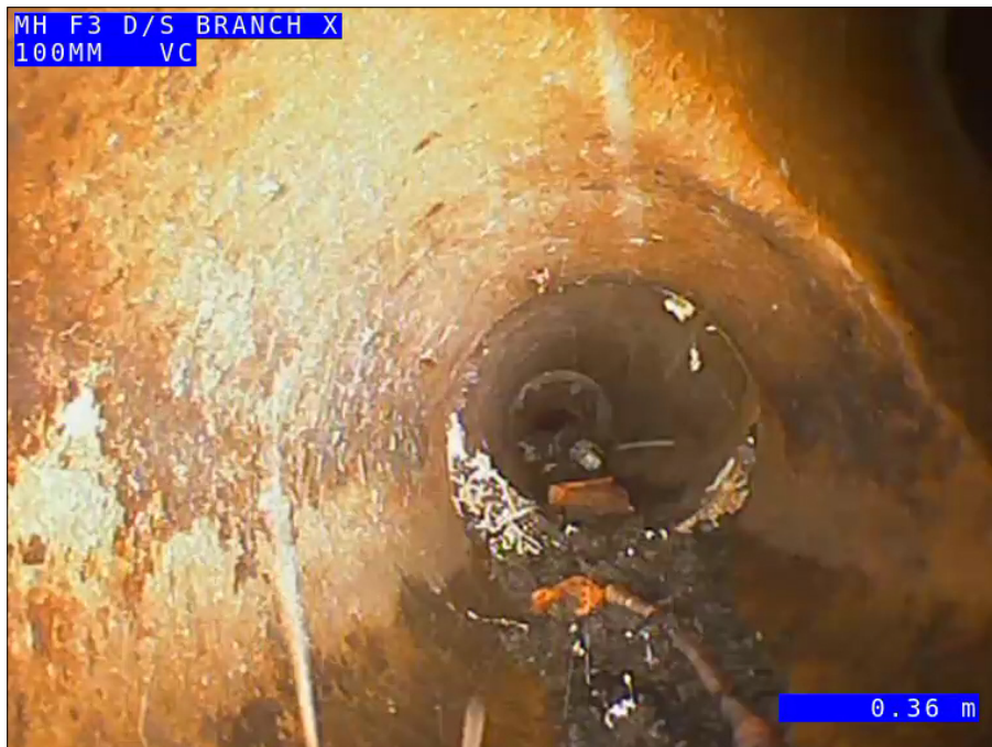
Photo: 16_16_98_A.jpg 0.36m, Junction, at 3 o'clock, diameter 100mm
