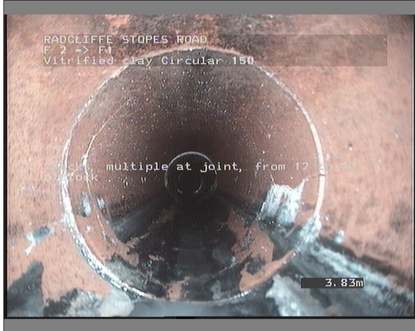
Photo: 15_15_85_A.JPG 3.83m, Cracks, multiple at joint, from 12 to 12 o'clock
