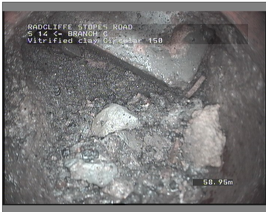
Photo: 7_7_31_A.JPG 58.95m, Finish node type, other special chamber reference number: BRANCH C
