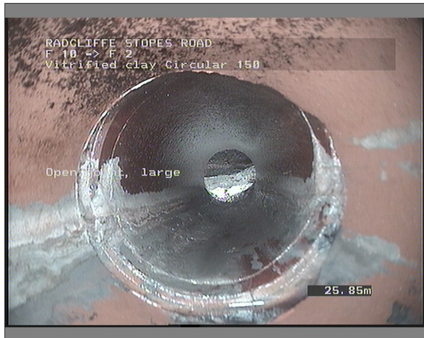
Photo: 12_12_73_A.JPG 25.85m, Open joint, large
