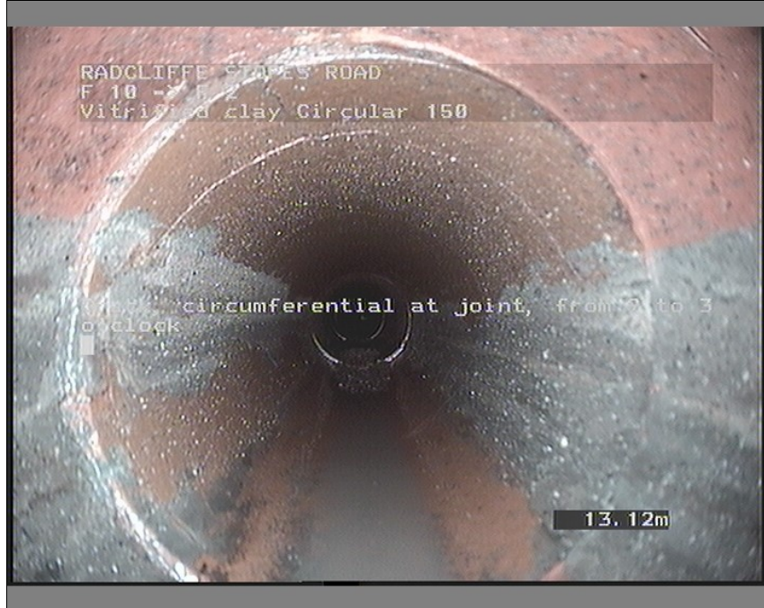
Photo: 12_12_68_A.JPG 13.12m, Crack, circumferential at joint, from 9 to 3 o'clock
