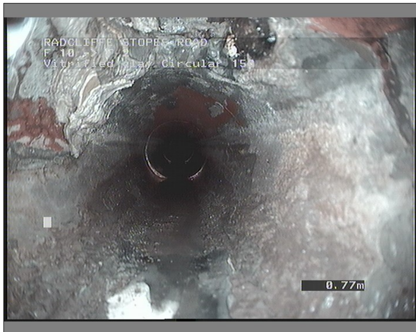
Photo: 12_12_63_A.JPG 0.77m, Connection other than junction, at 12 o'clock, diameter 100mm
