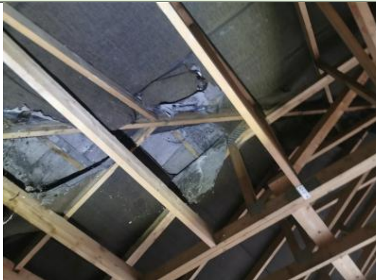
B2: Interior of B2, roofing felt gaps with cobwebbing
