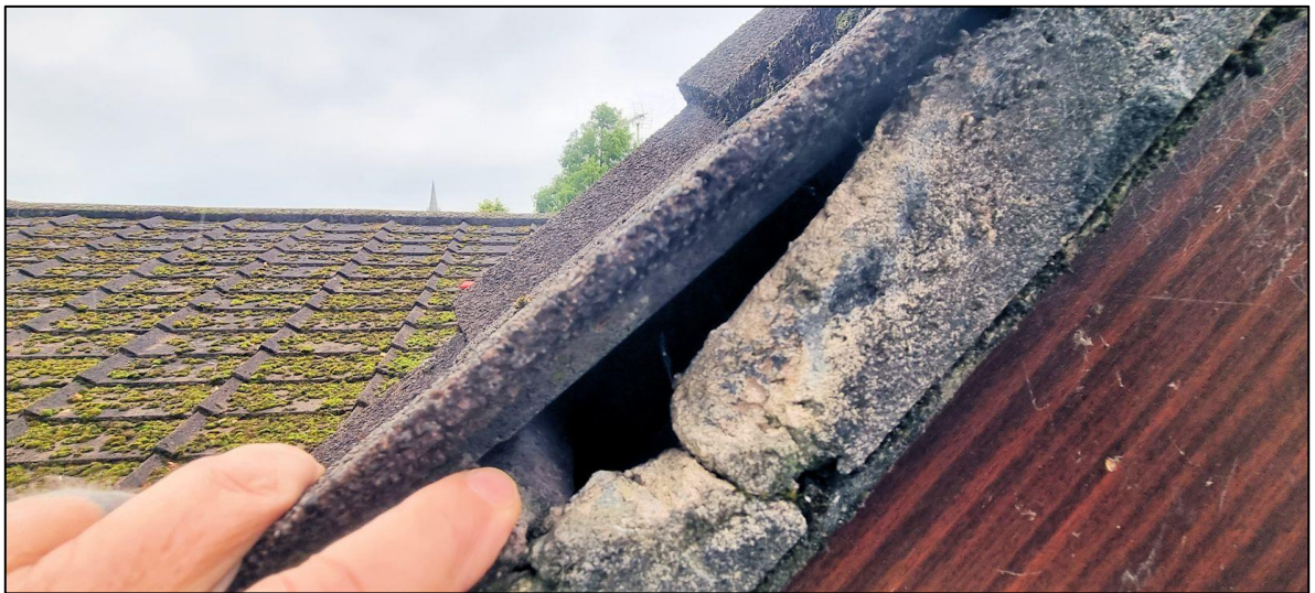
Plate 6: Missing mortar in the verges opened to extensive spaces under the tiles.
