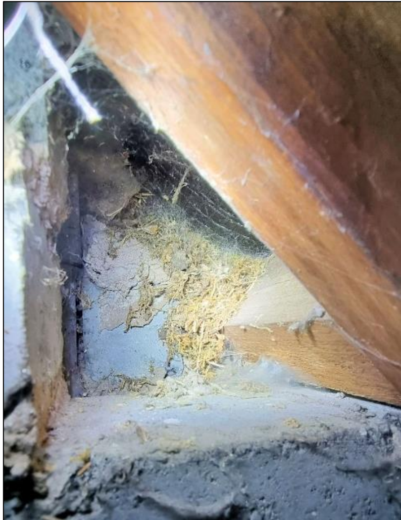
Plate 21: Evidence of nesting in the void above the garage.
