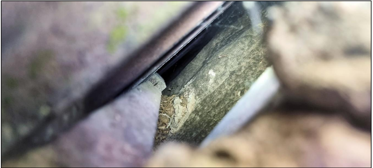
Plate 7: The gaps in the verges led to extensive spaces under the roof pitches that were not suitable for roosting crevice dwelling bats.
