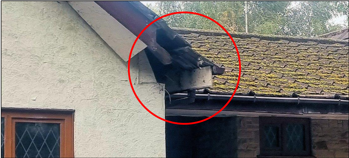
Plate 9: Recently damaged barge boards and soffits were noted but were not considered to offer any roosting potential.
