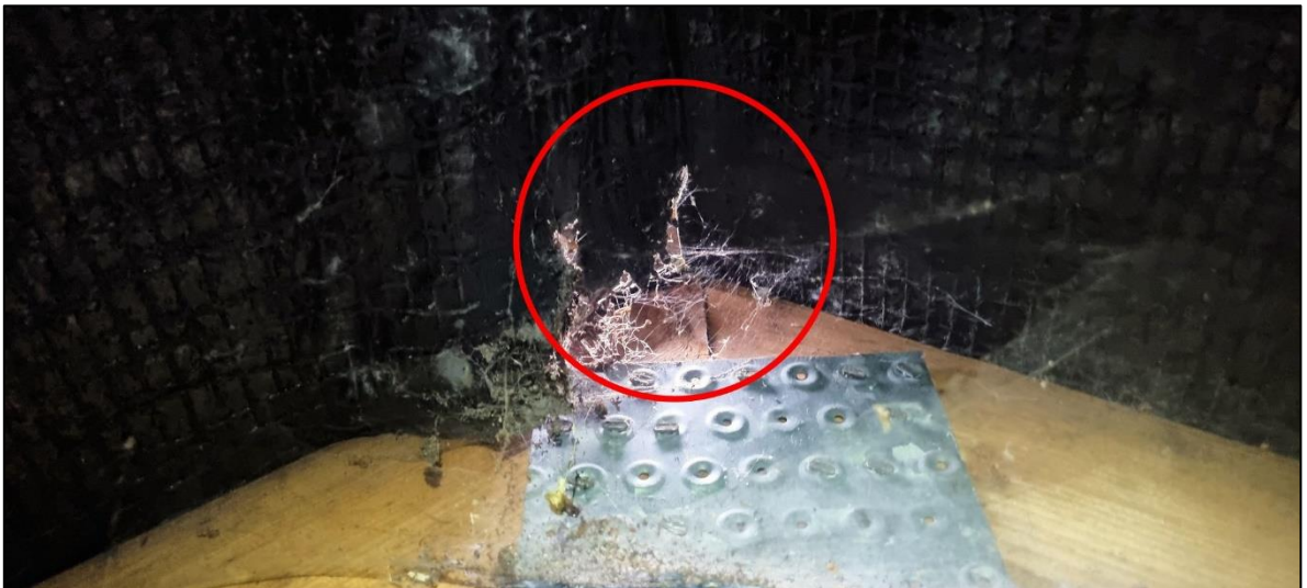
Plate 16: In some places along the ridge, the membranes were damaged but these did not gave any potential access to the internal void.
