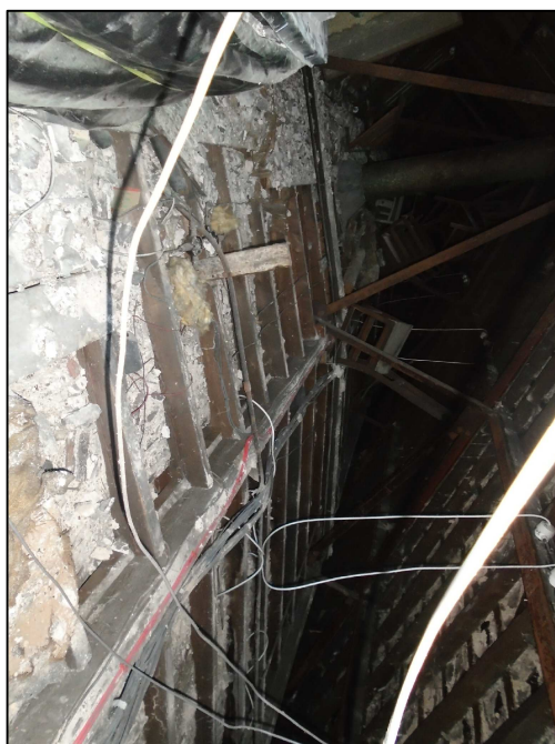
PHOTO 7 : MAIN ROOF LOFT SPACE Showing detritus in it ( to be cleared )
