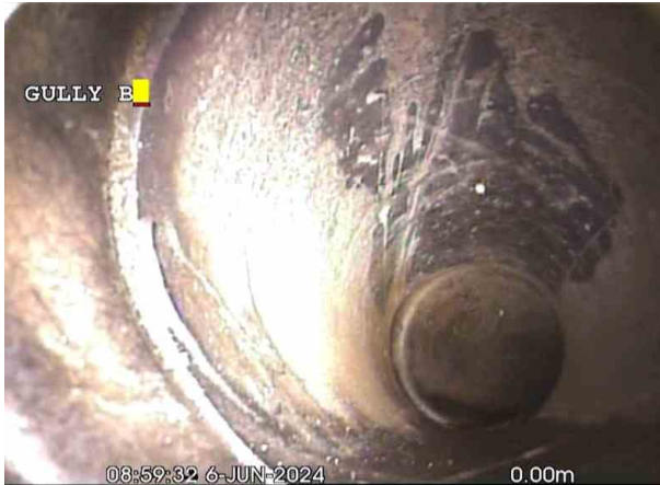
GULLY BX_62f342fd-36d7-446f-affd-e7fb434d18b6_20240606_13013 7_393.jpg, 00:00:00, 0.00 m General photograph taken at this point
