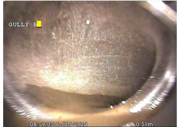
GULLY BX_9d17f683-b9d7-482b-b9dc-d7c99259cbd4_20240606_130 150_613.jpg, 00:00:03, 0.51 m Line deviates right, SLIGHT
