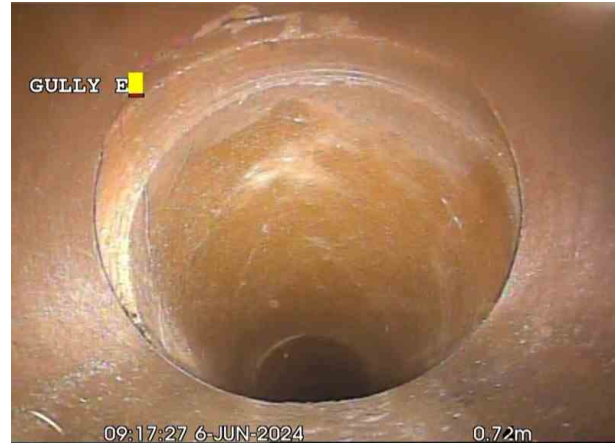
GULLY EX_fbda313f-64ec-4726-b4be-b0d7f1e4c4aa_20240606_130 736_835.jpg, 00:00:05, 0.72 m Joint displaced, medium, WHERE LINE IS DROPPING DOWN TO MIAN
