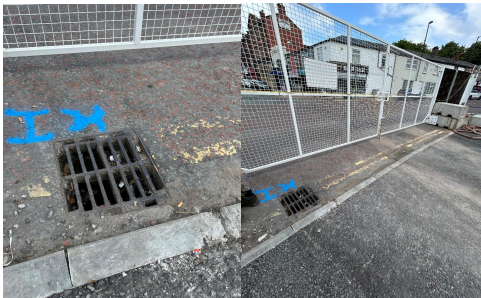
GULLY I AND ITS LOCATION
