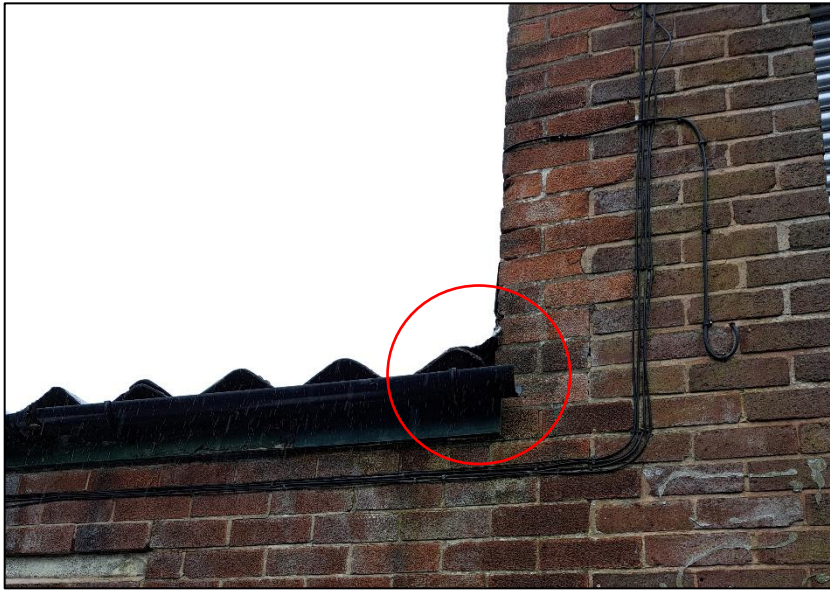
Photograph 4 showing gap beneath corrugated roof and lead flashing
