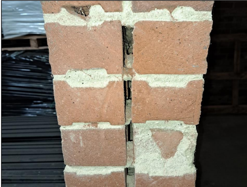
Photograph 10 showing cracks in walls between rooms
