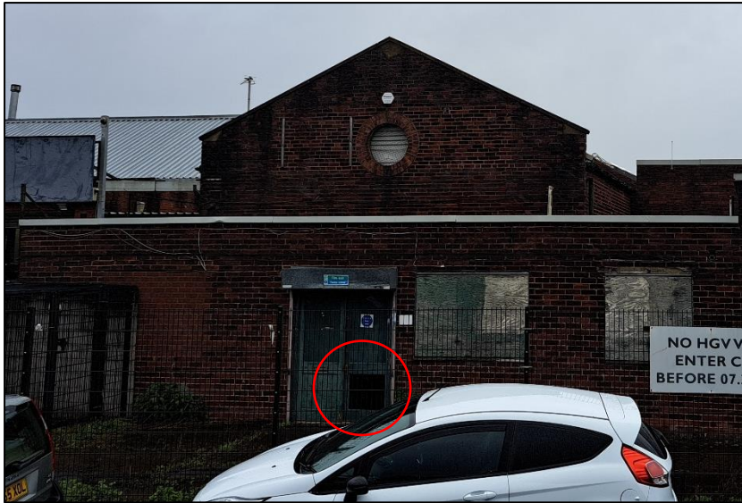
Photograph 2 showing front of the property and the gap in the door
