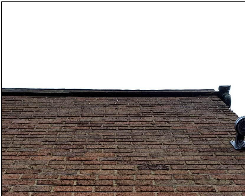
Photograph 5 showing gap at fascia
