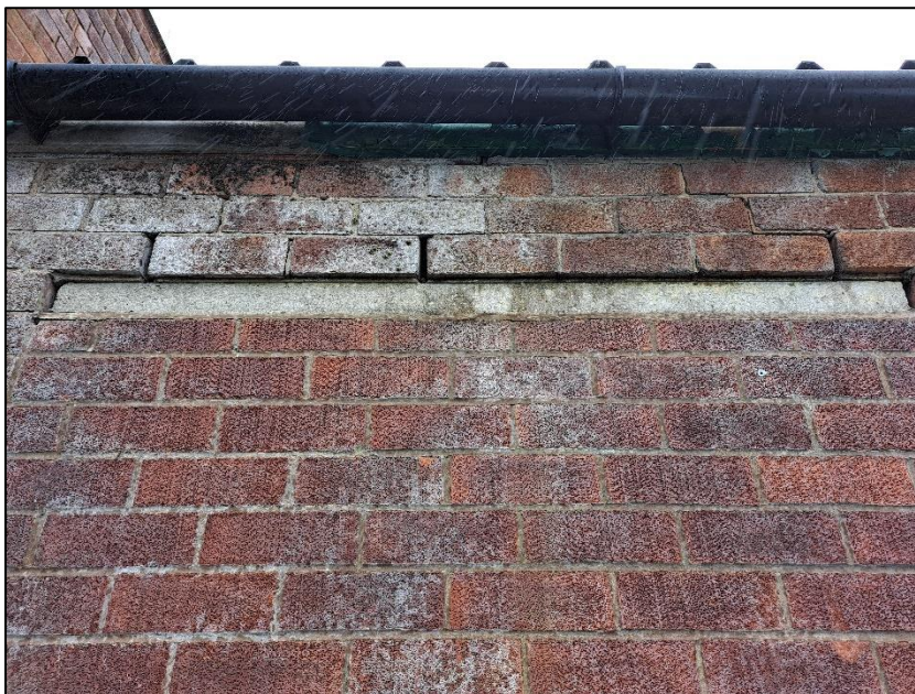
Photograph 3 showing gaps in the masonry from the side elevation
