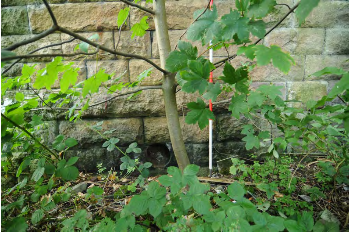
Photograph No : 75 Digital Ref: HOMI_HBR_0022 Direction: SW Description: Opening in lower stone course in north elevation of Building C
