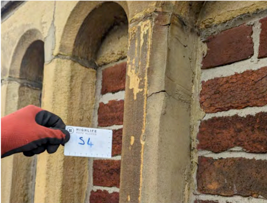
Photo 5 – Previous mortar repair to upper section of stone mullion ( extract Highlife Rope Access Report )
