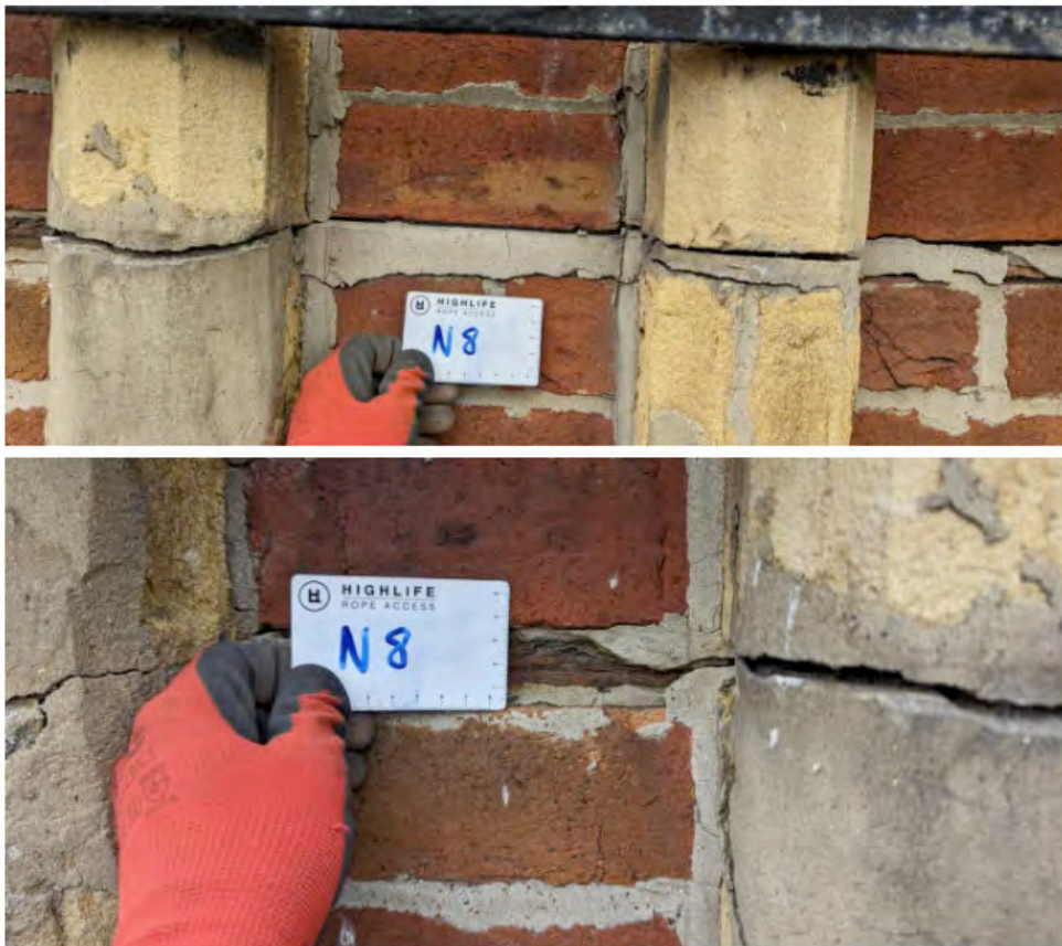
Photo 3 – Significant corrosion to embedded iron band in mortar joint (extract Highlife Rope Access Report )
