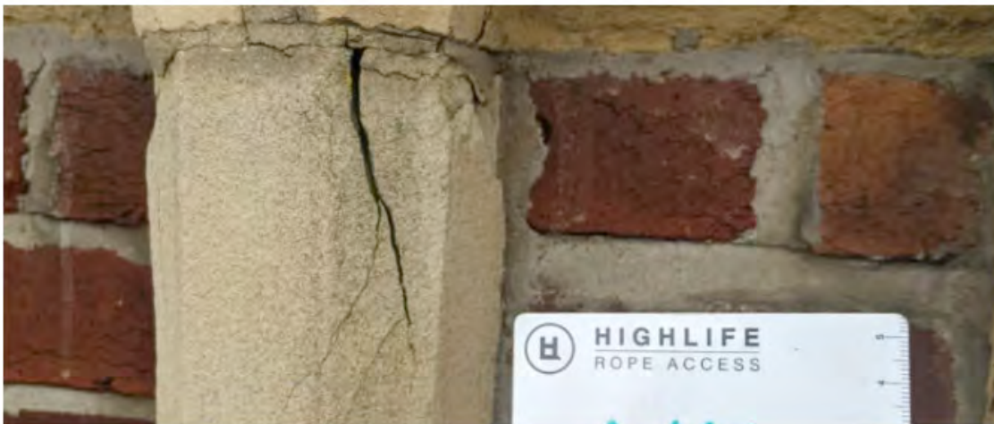
Photo 6 – Diagonal fracture in upper section of stone mullion, likely from corroding ferrous fixing ( extract Highlife Rope Access Report )
