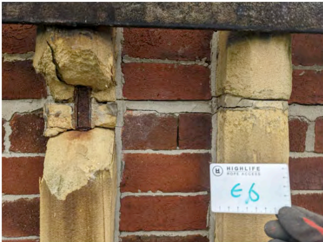
Photo 4 – Significant corrosion to ferrous dowel between stone mullions (extract Highlife Rope Access Report )
