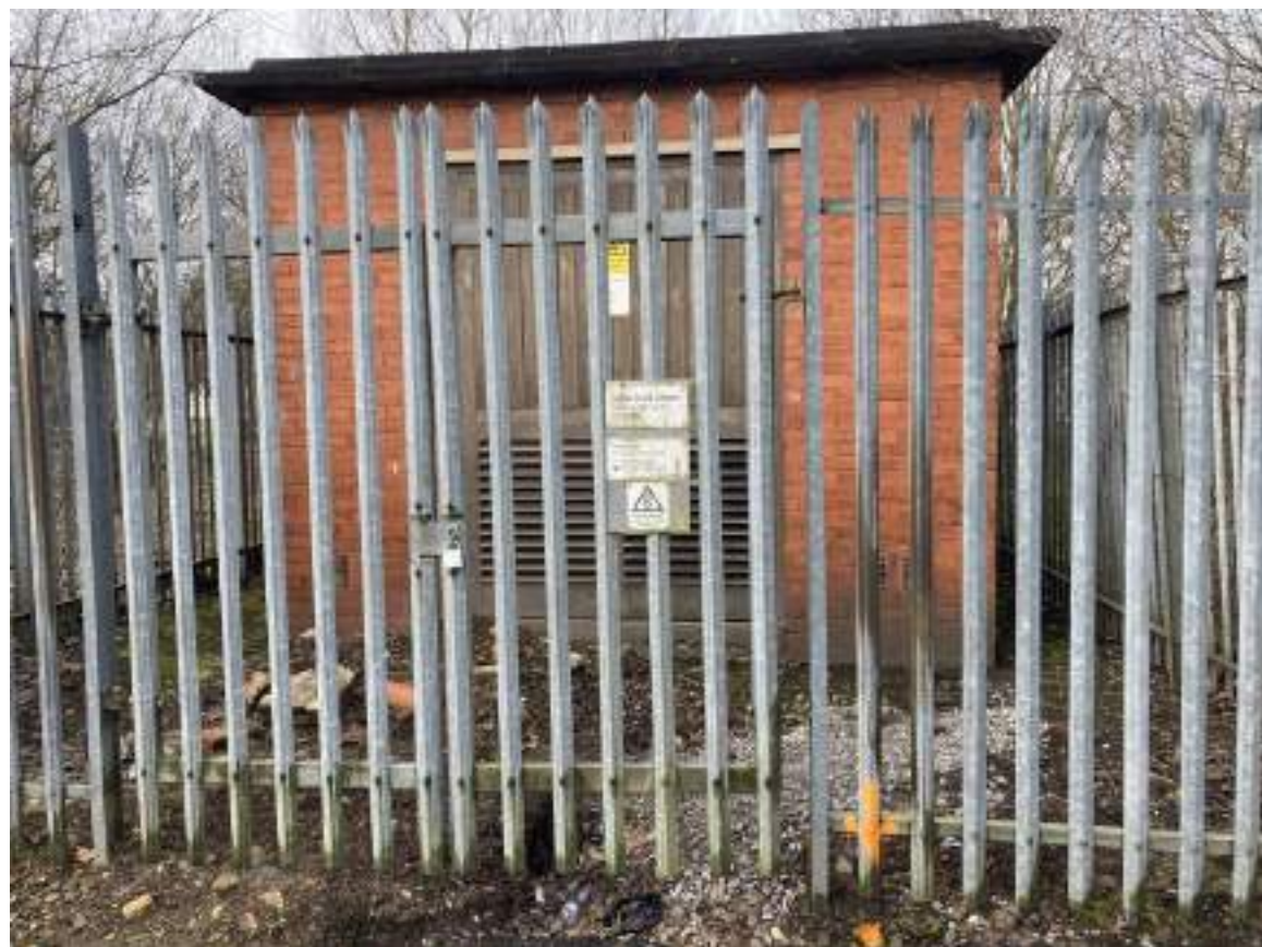
Plate 15 – Electrical substation in north west corner
