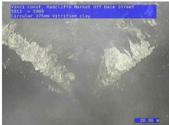
20.06m – Encrustacion (20% cross section loss)
