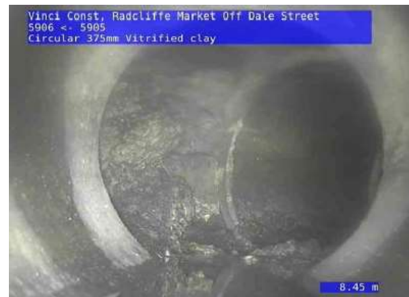
41.89m – Settled deposits, 15% cross sectional area
