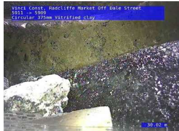
30.02m – Encrustacion (20% cross section loss)
