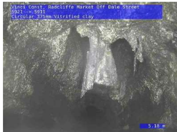
5.18 – attached deposits (encrustation)
