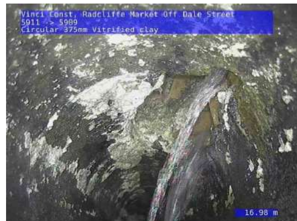
16.98m – defective connection (part blocked)
