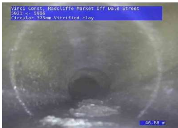
46.86 – Hard or compacted settled deposits
