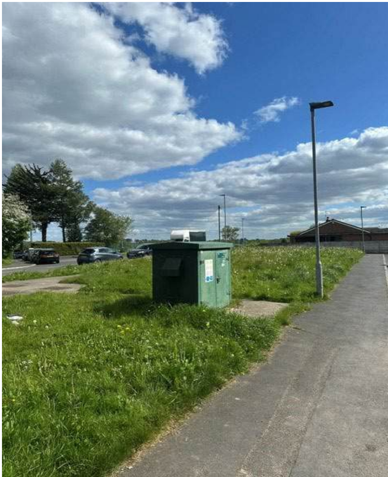
Photograph 5: View of the United Utilities kiosk, located adjacent to the northern Site boundary, facing south west (showing the Site area to the rear of the kiosk)
