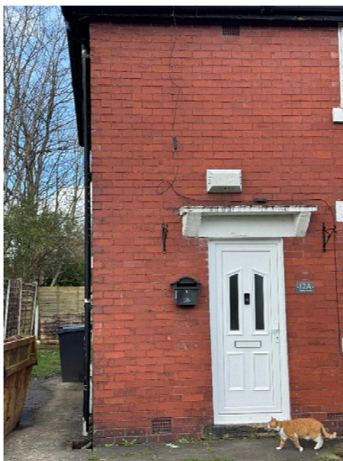
Front Elevation wall outer plumbness
