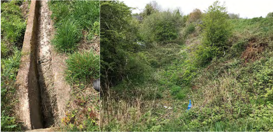
Photographs 1 and 2 – showing the high-level overflow and low-level drain-down valve
