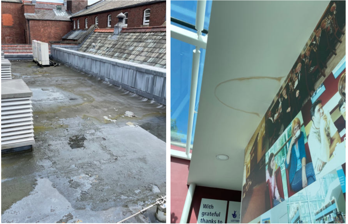
05 (Area F). Evidence of ponding to the flat roof, extensive coating failure and patching. Right, internal water ingress and damage to finishes.
