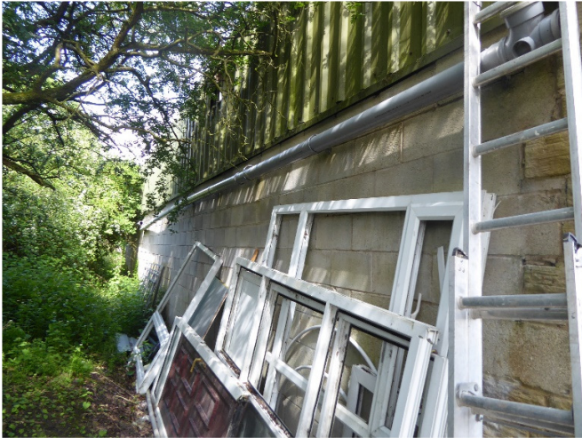
SW elevation: Localised gaps between masonry wall plate / upper steel section walls, leading to wall cavity. Area is very 'cluttered' by adjacent tall mature hedge close to building.
