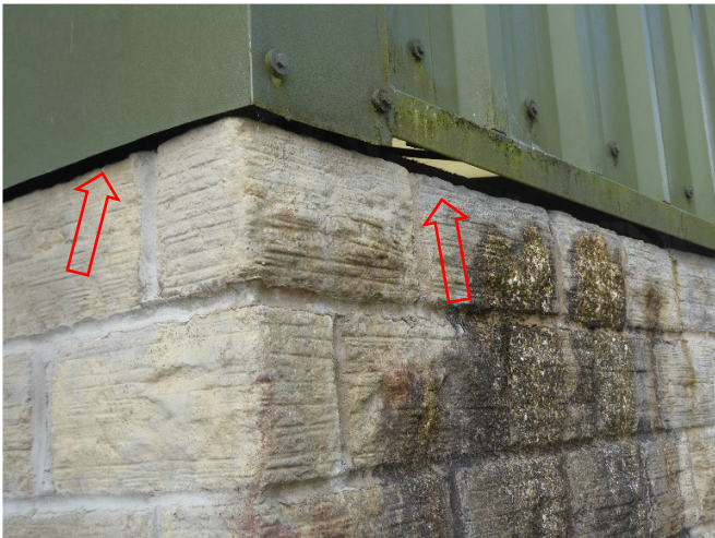
NE / NW elevation corner: Gaps between masonry wall plate and upper steel section walls, leading to wall cavity.
