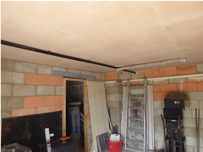
SE end of building where the ceiling is plaster boarded without any access to the roof void / loft.
