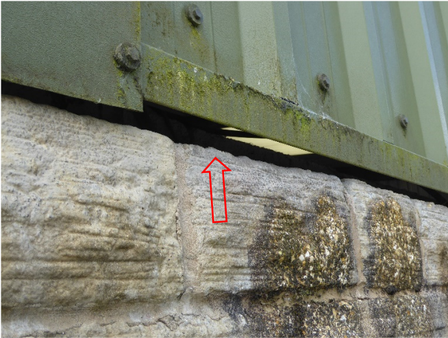
NW elevation: Gaps between masonry wall plate and upper steel section walls, leading to wall cavity.
