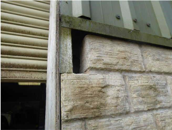
NE elevation: Hole in masonry leading to wall cavity.
