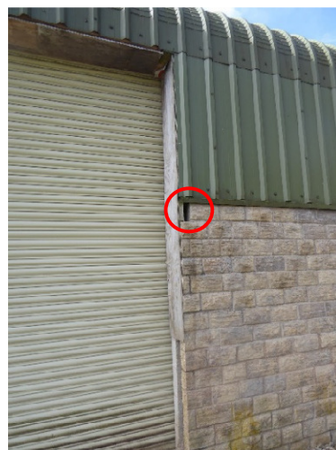
NE elevation: Hole in masonry leading to wall cavity.
