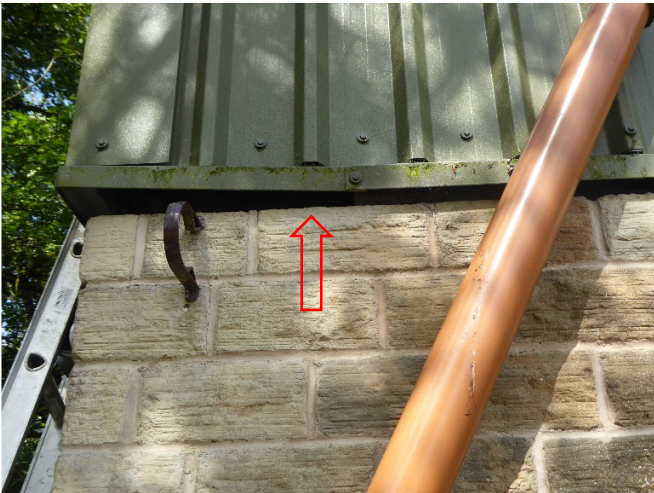
SE elevation corner: Gaps between masonry wall plate and upper steel section walls, leading to wall cavity.
