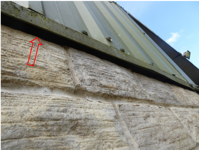
NE elevation: Continuous gap between masonry wall plate and upper steel section walls, leading to wall cavity.
