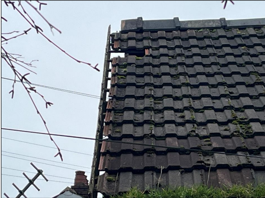
Plate 1 – Degradation on the eastern side of the clay-tiled roof
