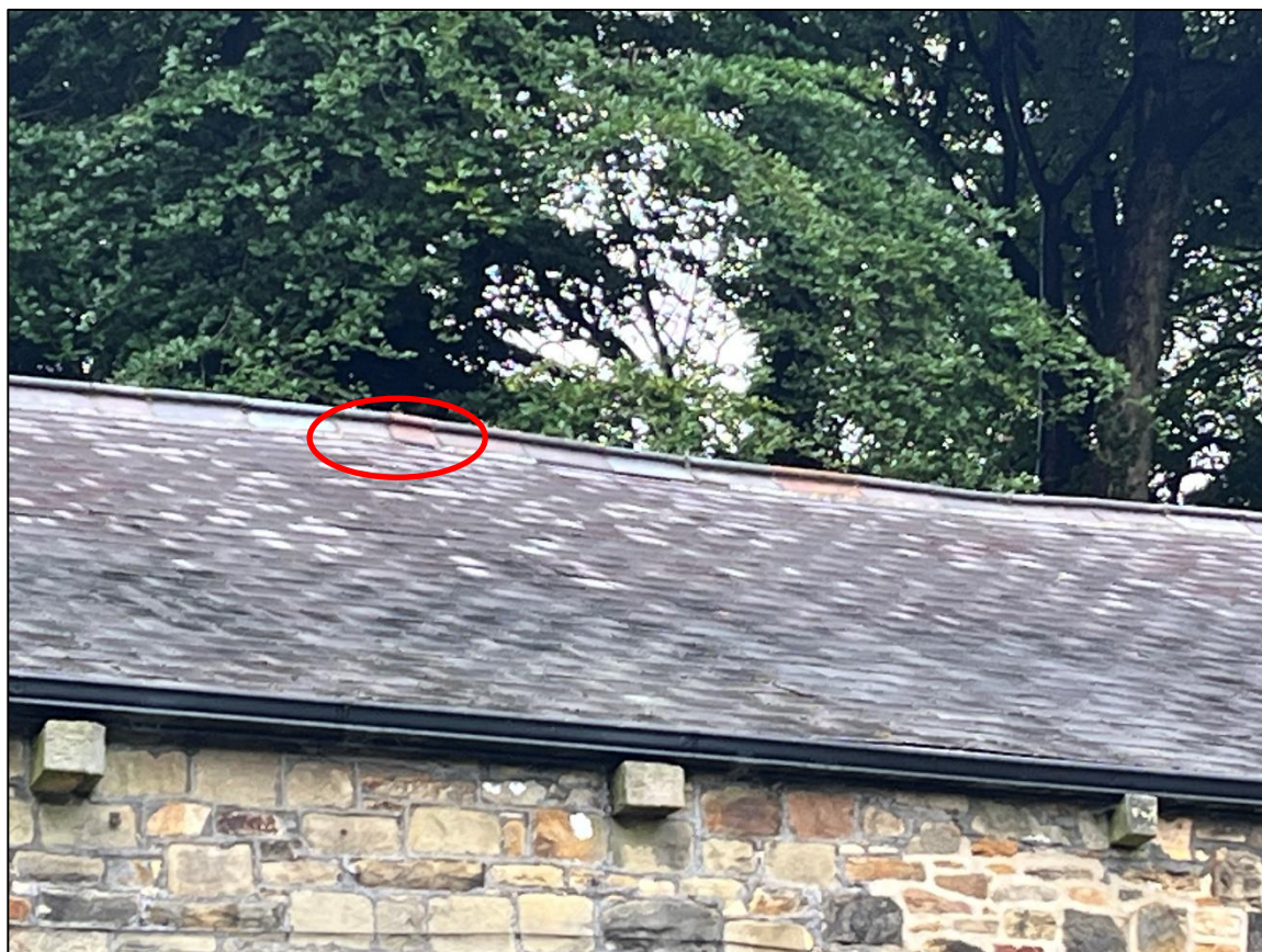
Plate 7 – Example of gaps beneath ridge tiles
